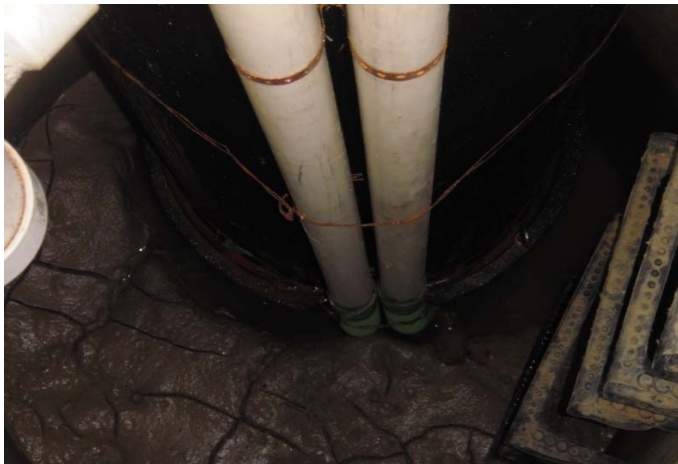
Picture 305- Pooled water below the eductor head was noted within two (2) of the DDC wells.
