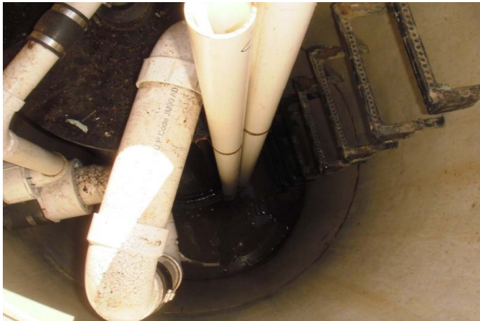
Picture 385- Groundwater observed on floor of three (3) DDC vaults.
