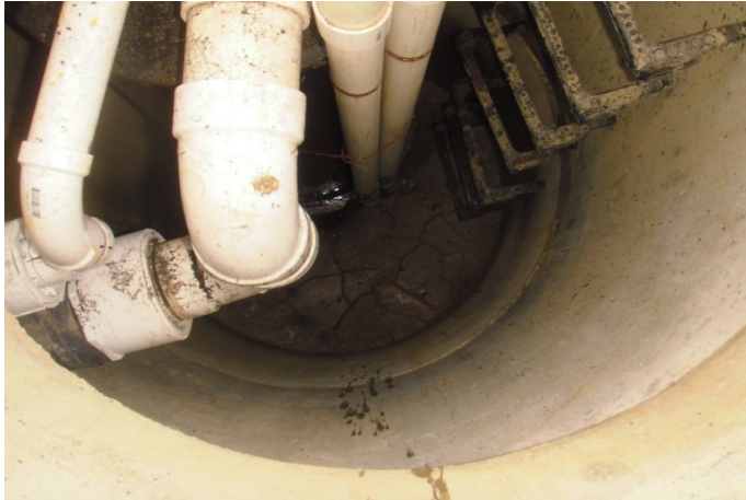
Picture 305- Some groundwater noted on vault floor beneath eductor for several DDC wells.
