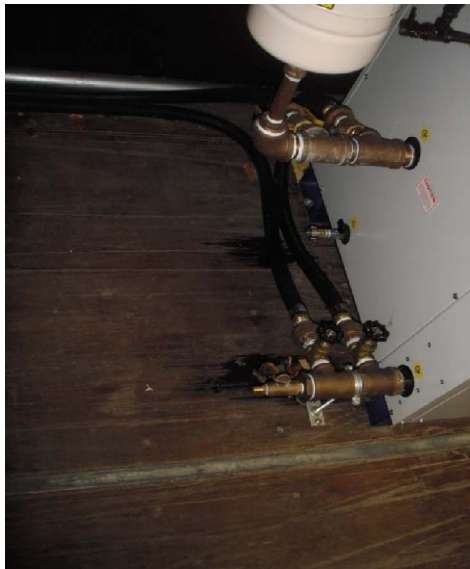
Picture 307- Minor pooled water was noted on the valve and hose beneath the chiller unit.
