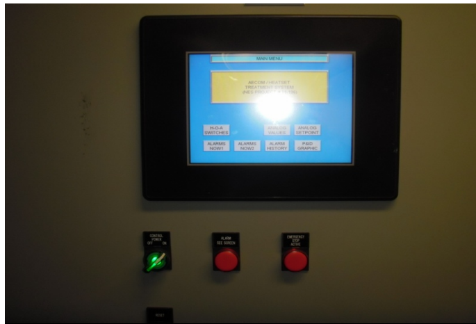
Picture 303- Both blower were up, with no alarms were triggered upon arrival.
