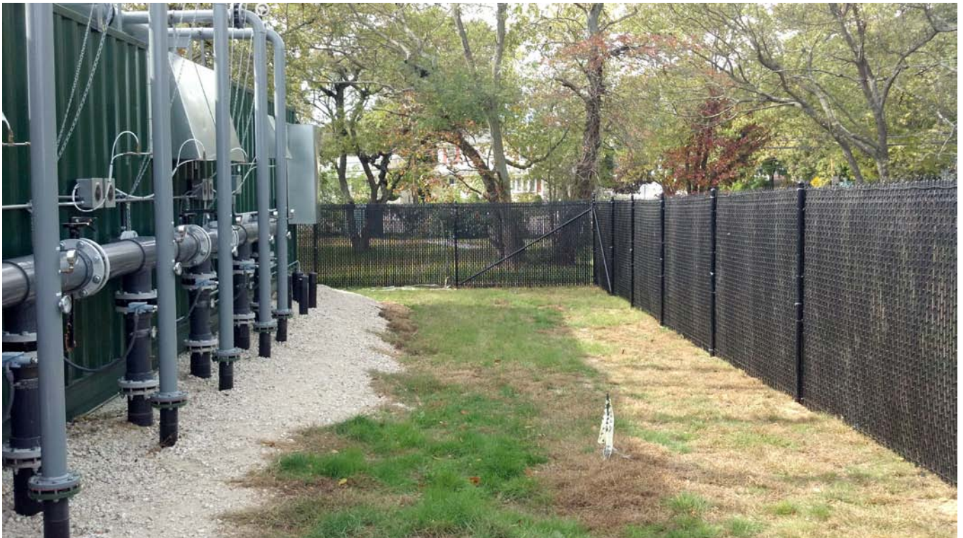
View of fencing along north side of treatment system pad.
