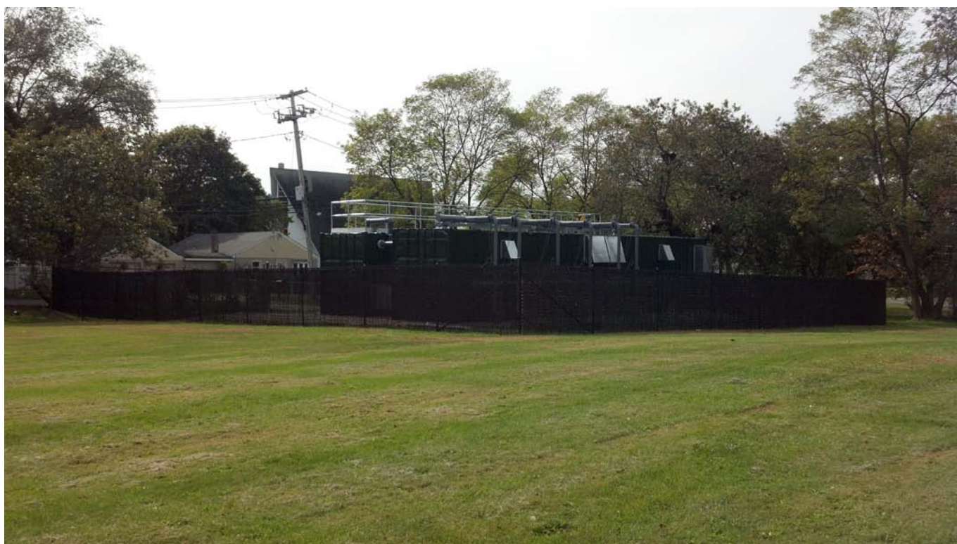
View of fencing around treatment system compound.
