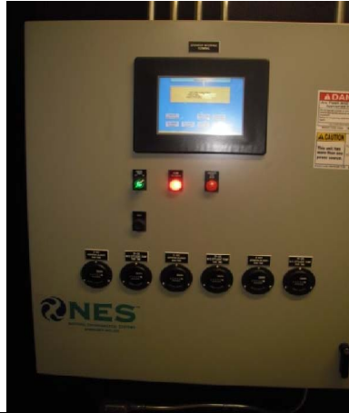
Picture 302- The "W9: Well DDC-10 Low Differential Pressure" alarm was triggered on the control panel upon arrival.
