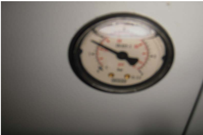
Picture 303- The chiller unit pump pressure gauge read 25 PSI.
