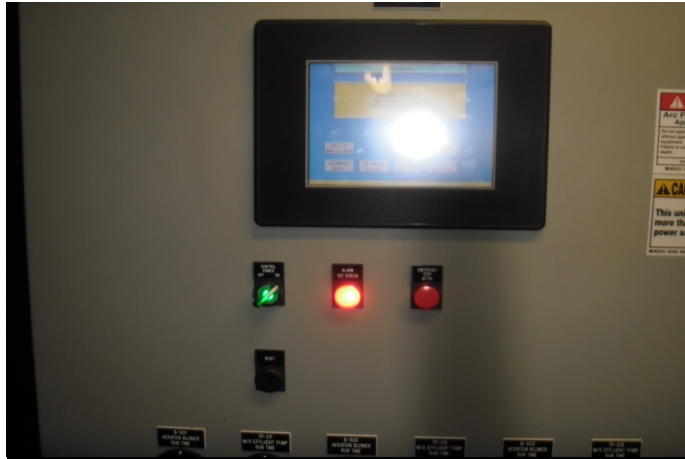
Picture 302- System was "Up" upon arrival with three (3) alarms triggered.
