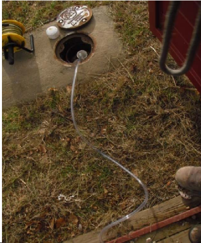
Picture 367- DDC-5 & DDC-6 condensate drainage valves were drained for 15 minutes.
