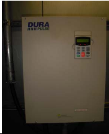
Picture 381 - The variable frequency drive (VFD) for System #2 was replaced on January 16th, 2013 by D&D electric.
