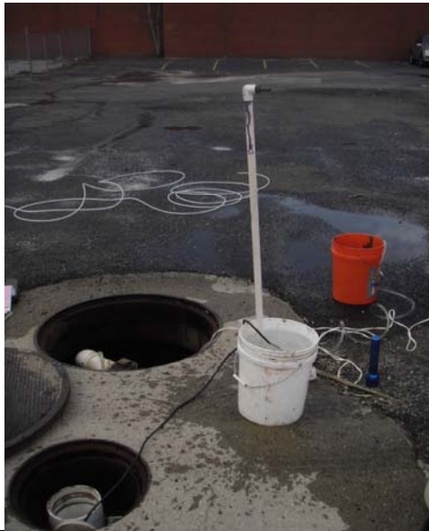
Picture 396 - The sump pump associated with DDC-4 was taken out and tested within a 5-gallon bucket of water. Pump was determined to be non-functioning and needs to be replaced.
