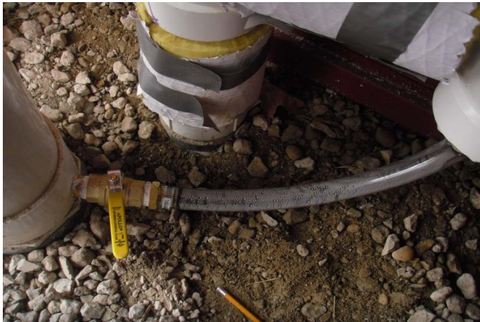
Picture 462- The one (1)-inch condensate line was observed no pooled water.
