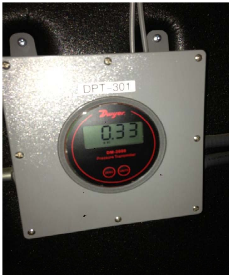
Picture 3578- Differential pressure gauge, DPT-301, read .33 IWC.
