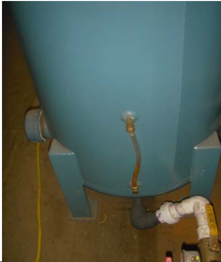
Picture P5090068 - No water was detected within the site glass of the knock-out tank.
