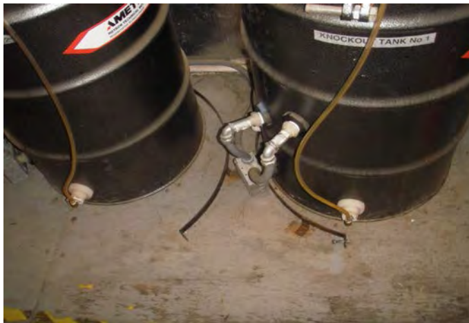
Picture P6060127 - Five (5) -inches of water was detected within the site glass of Knock-Out Tank No. 1 after adjusting the flow gauges associated with System #1.
