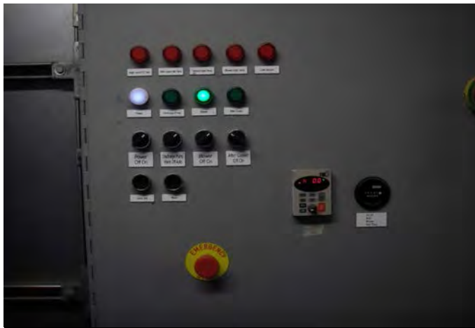
Picture P6060123 - Both systems were running with no alarms lit upon arrival.
