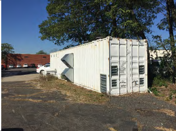
Onsite DDC System #2 Trailer
