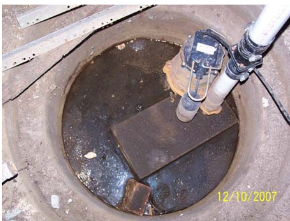
EC Site Sump in basement.
