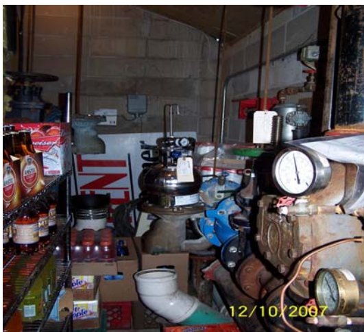
EC Structure 01 Sprinkler Room Air
