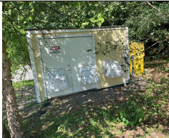
1. Oxygen Injection System.
