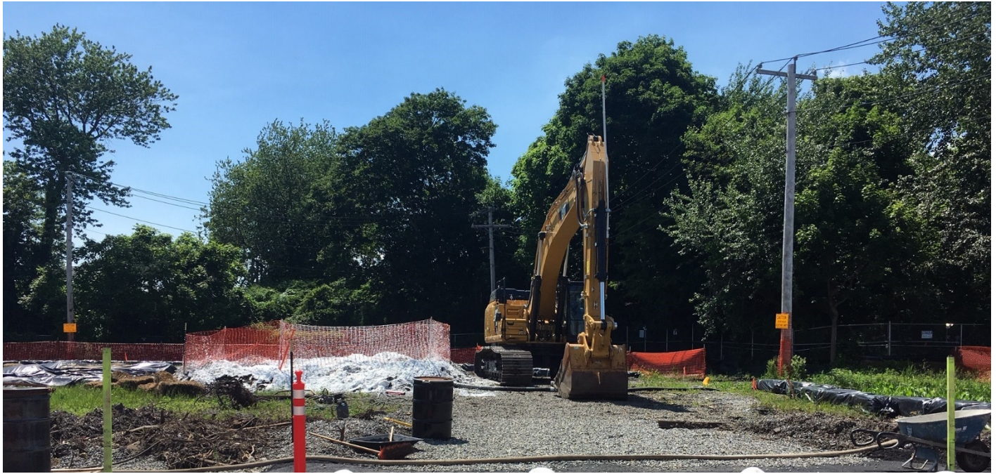
Photo 3: Pilot test area at end of work day. Excavation area is fenced and covered with foam to prevent odors.
