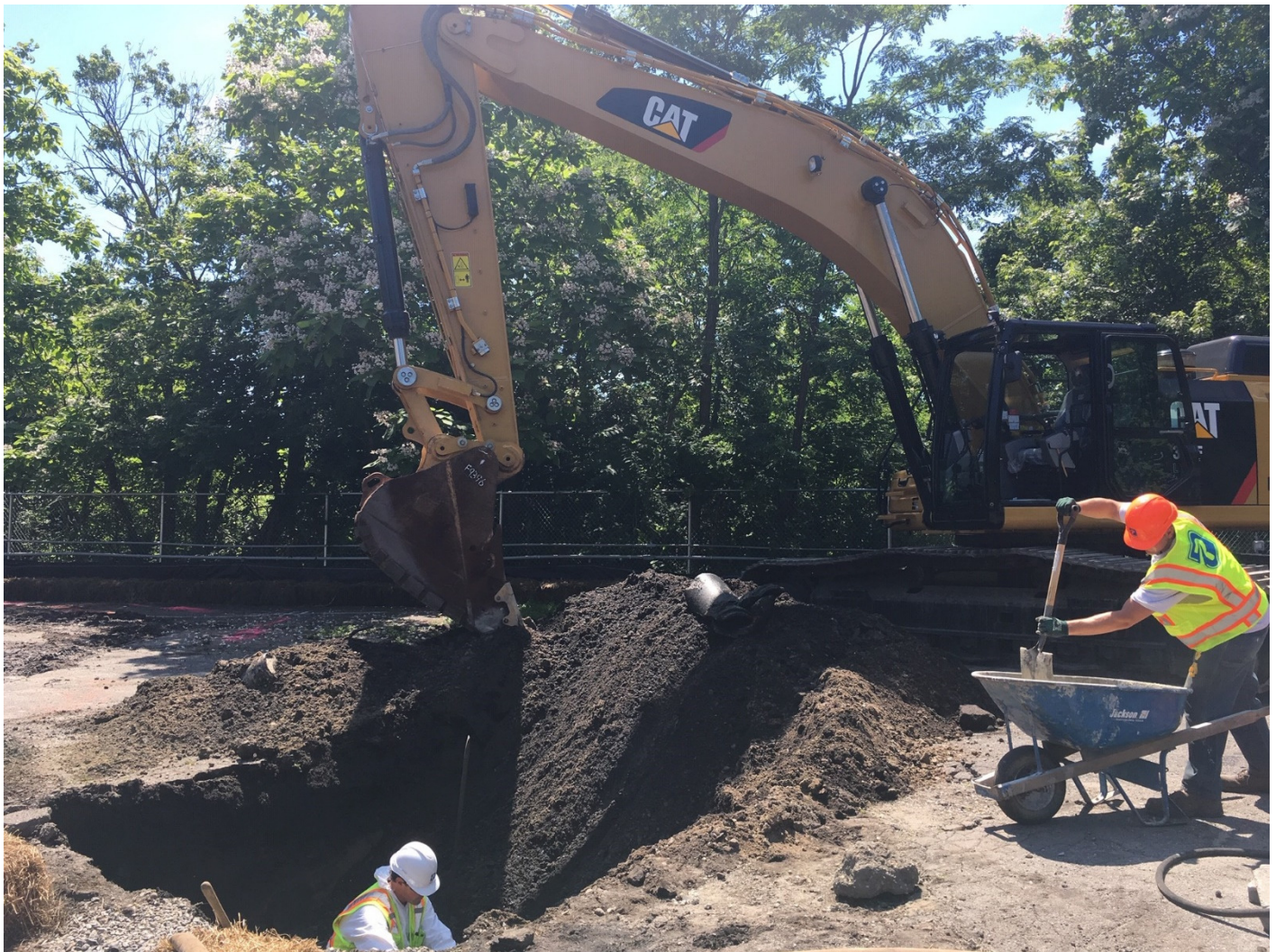
Photo 1: Plugging clay pipe outflowing from southern catch basin (located at the bottom left corner of the picture).
