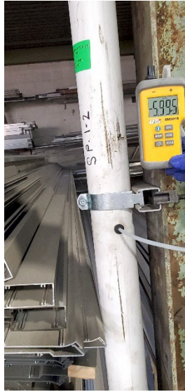
View of suction point, SP 1-2 and associated vacuum gauge with manometer reading.
