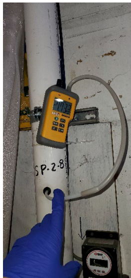
View of suction point, SP 2-8 and associated vacuum gauge with manometer reading.
