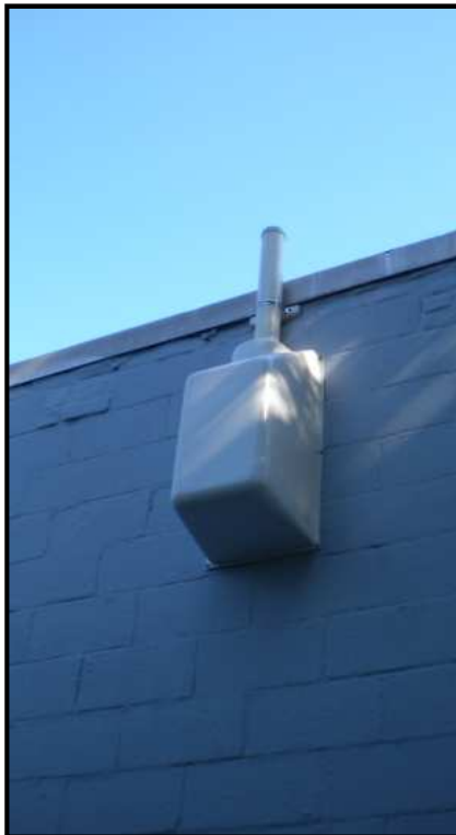
System 7 - fan and discharge piping
