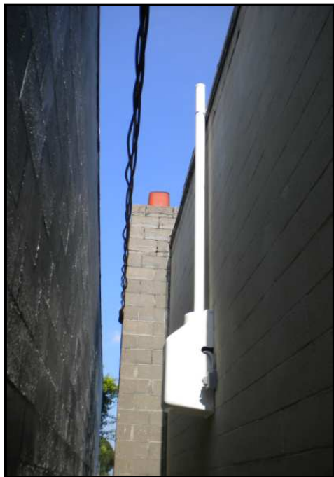
System 1 - fan and discharge piping
