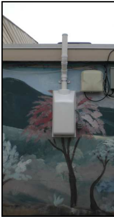
System 8 - fan and discharge piping
