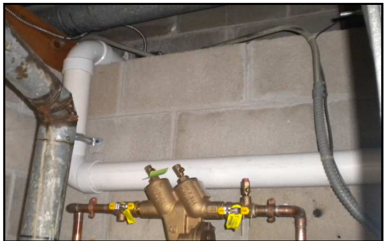
System 5 - interior piping
