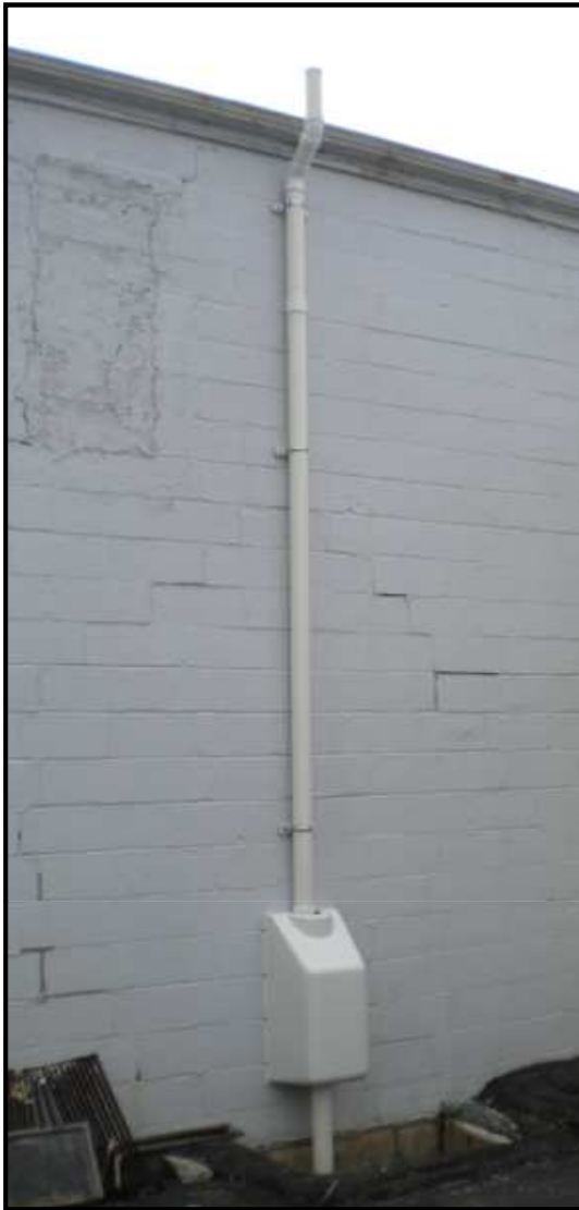
System 9 - fan and discharge piping
