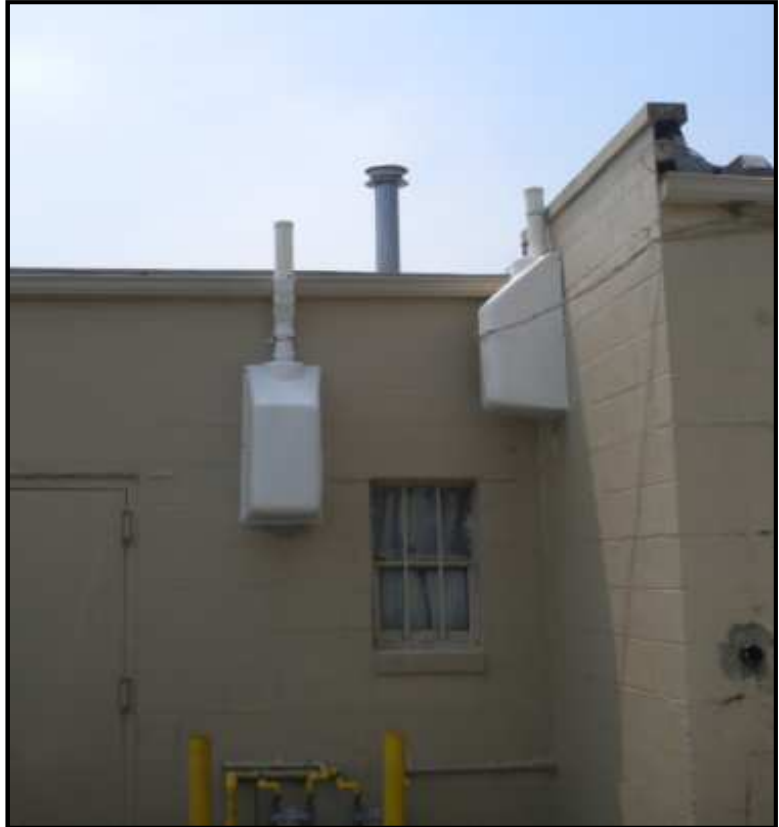
Systems 5 and 6 - fan and discharge piping
