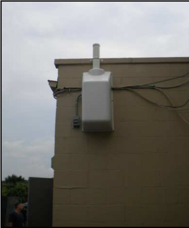
System 2 - fan and discharge piping
