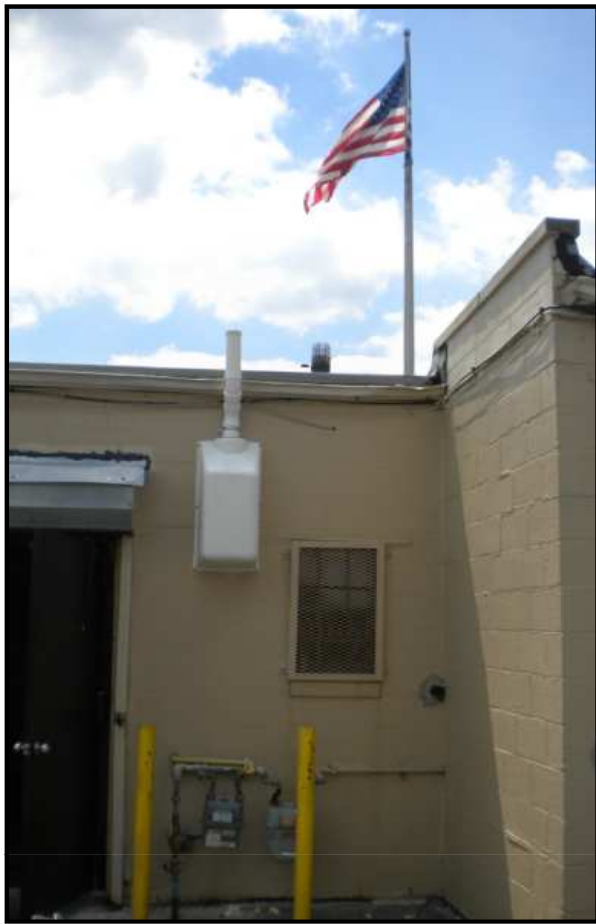
System 4 - fan and discharge piping
