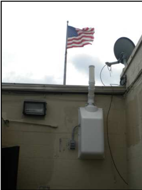
System 3 - fan and discharge piping
