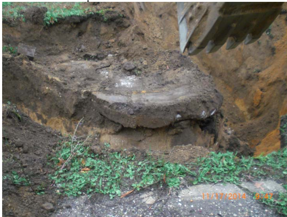
Photo 3: CP-5 Lid Exposed
