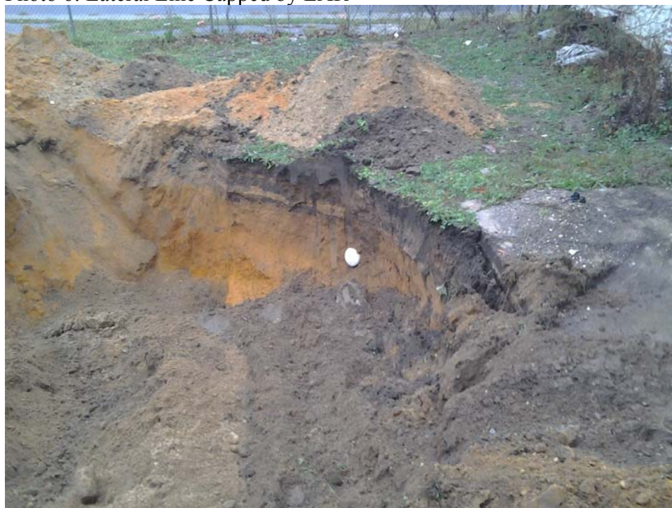
Photo 6: Lateral Line Capped by EAR
