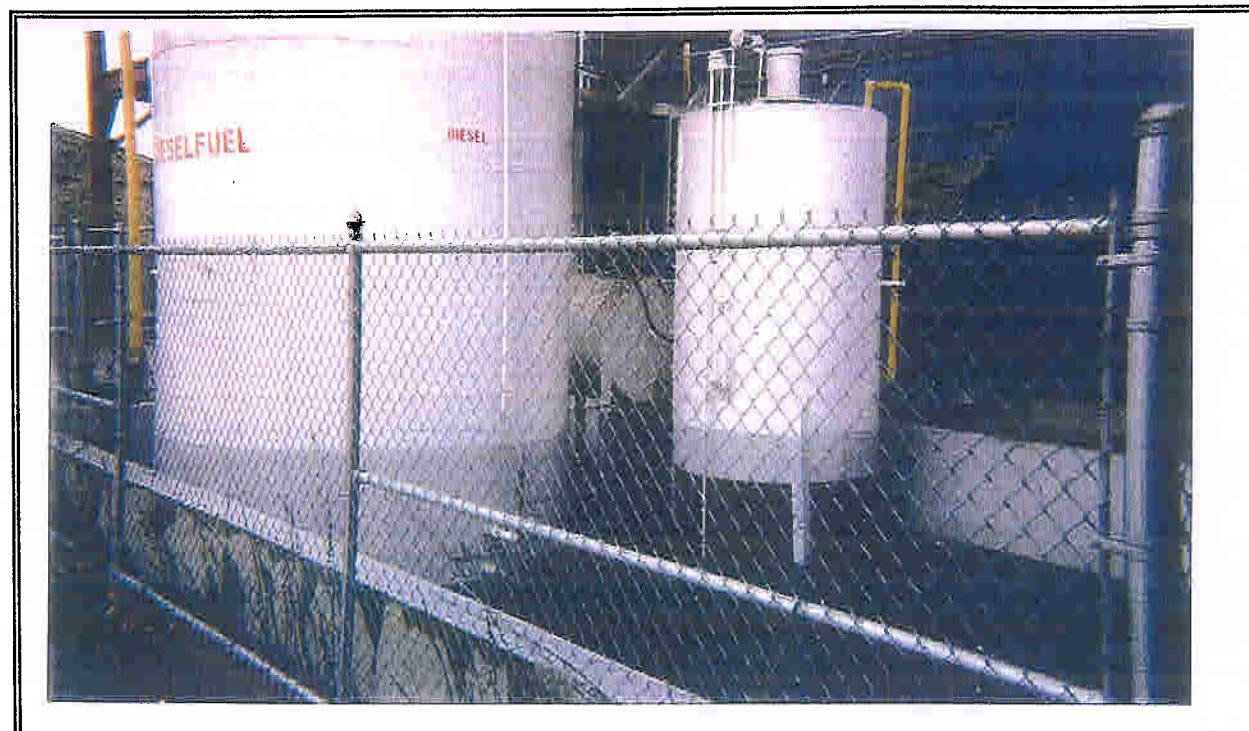
PHOTO 08: View of AST's and spill confinement barrier.
