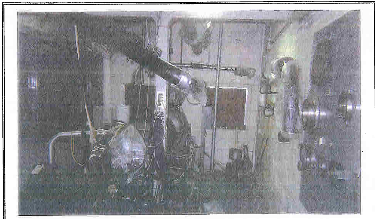
PHOTO 24: View of test cell.
