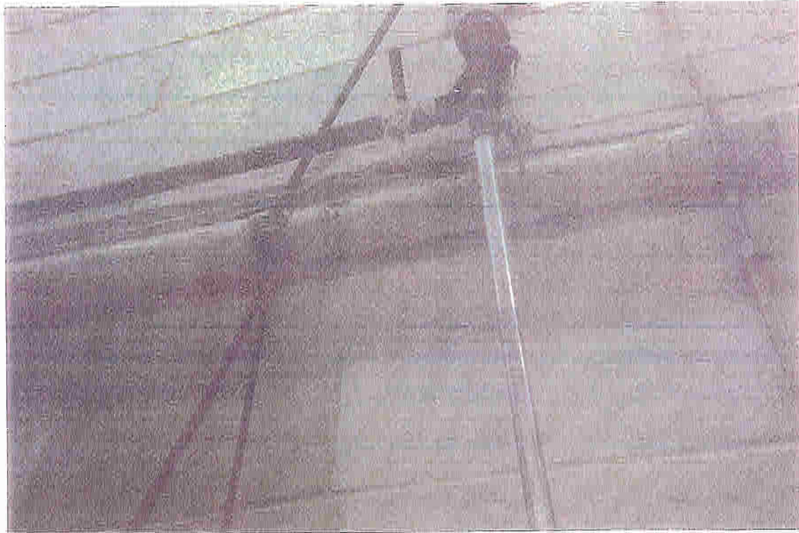
PHOTO 15: View of pipe insulation wrap.
