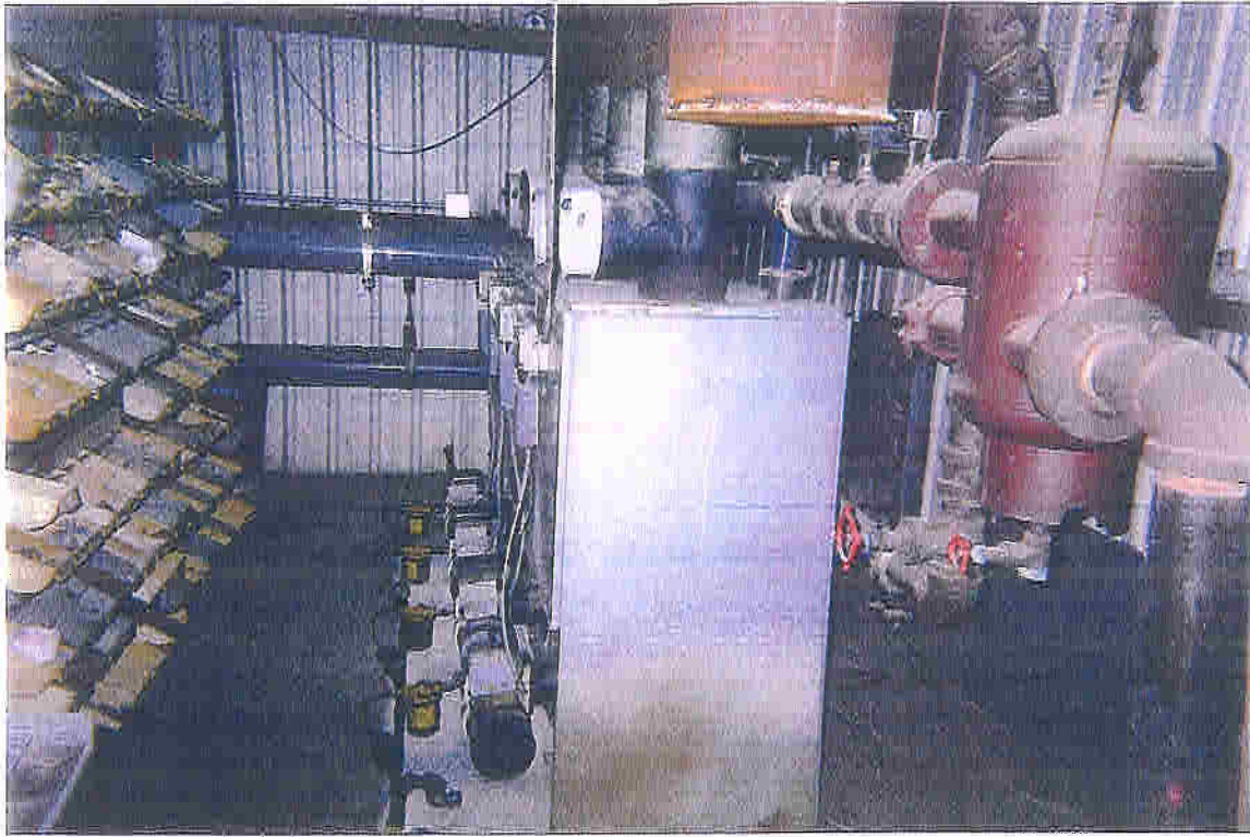
PHOTO 17: View of second story boiler room located in production area.
