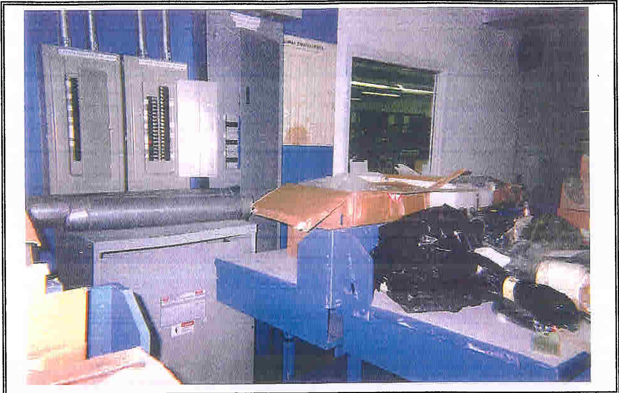
PHOTO 13: View of floor mounted transformer.
