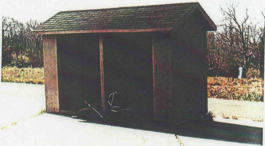
Deteriorated bus-stop shelter.
