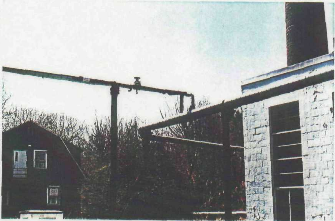
Central boiler room #P-105(on right) with exterior, asbestos-insulated pipes used for heating system. Bldg. #P-11 on left.
