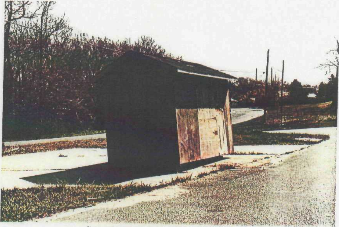
Deteriorated bus-stop shelter.
