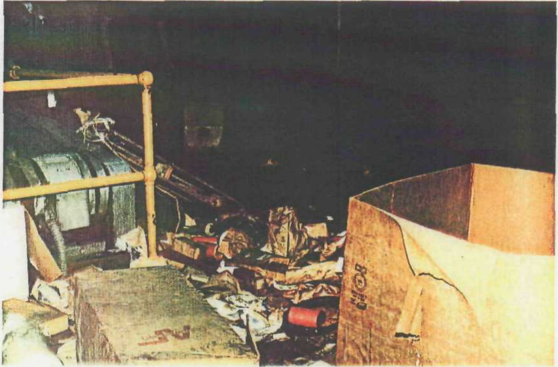
Vandalism in bldg. #P-203, Power House.
