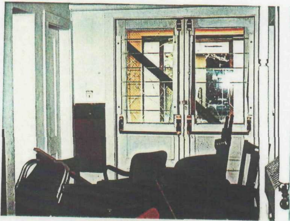
Vandalism in bldg. #P-9.
