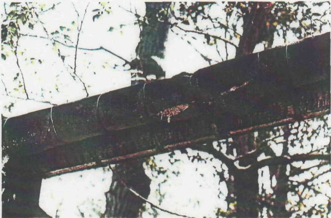
Asbestos-insulated pipes used for heating system with exposed asbestos leaking directly to the ground.
