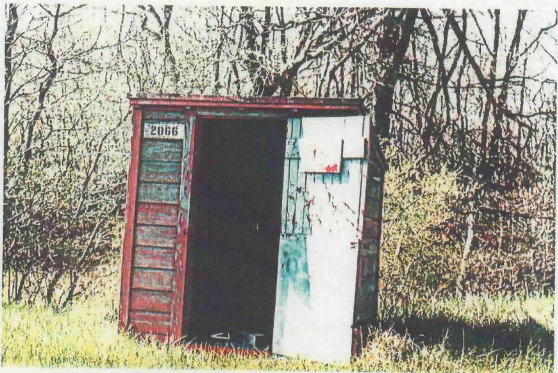
Deteriorated bldg. #2066 with fire hydrant (fire hydrant to be retained).
