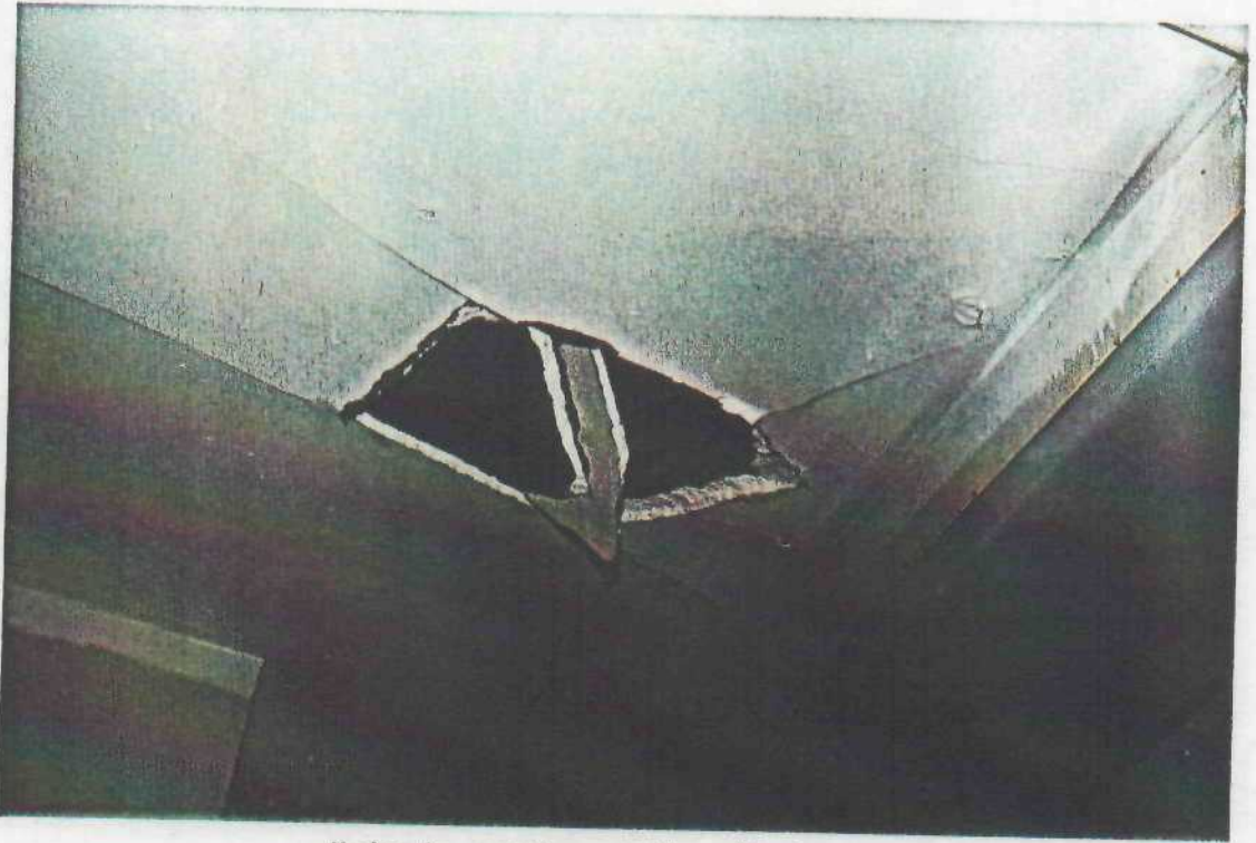
Hole in ceiling, bldg. #T-1.
