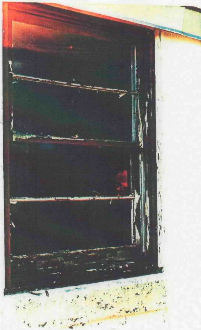
Broken glass in 2.5 foot high window of bldg. #P-119.
