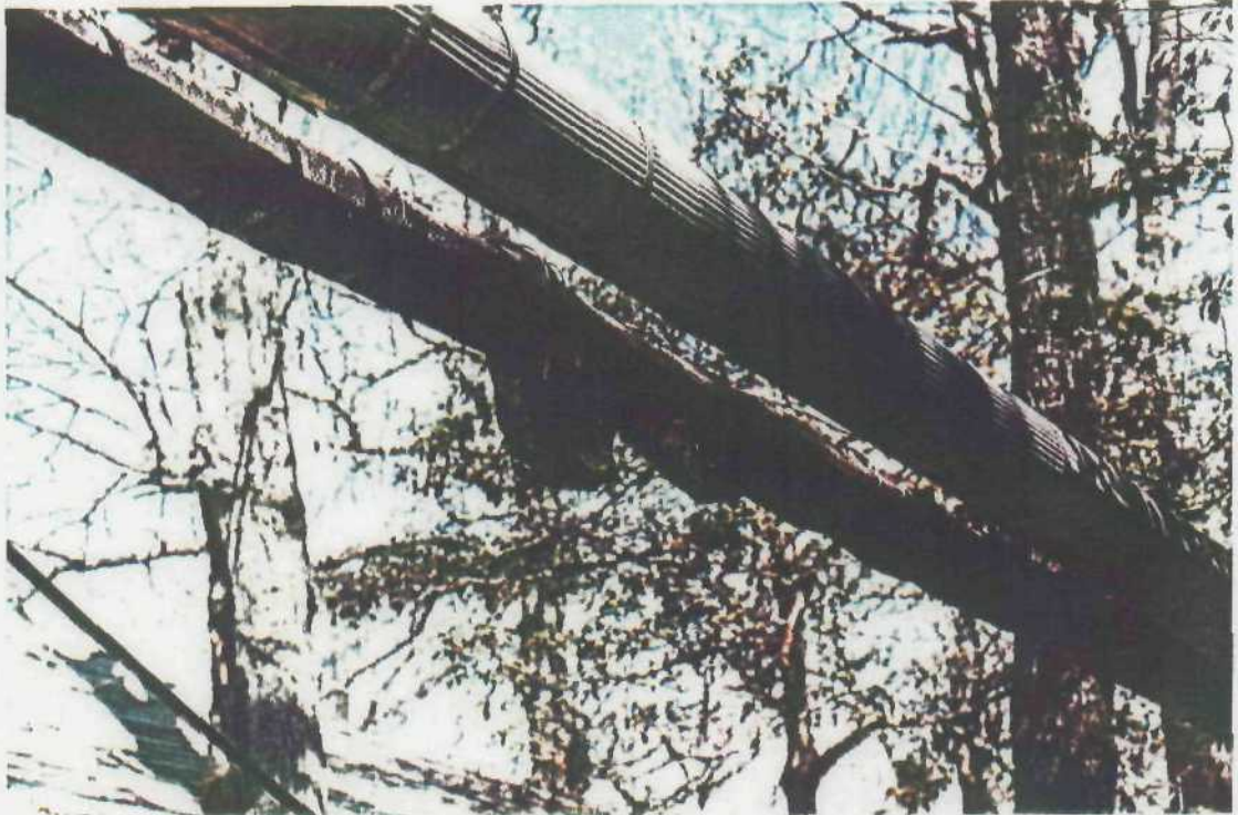
Asbestos-insulated pipes used for heating system with exposed asbestos is leaking directly to the ground.
