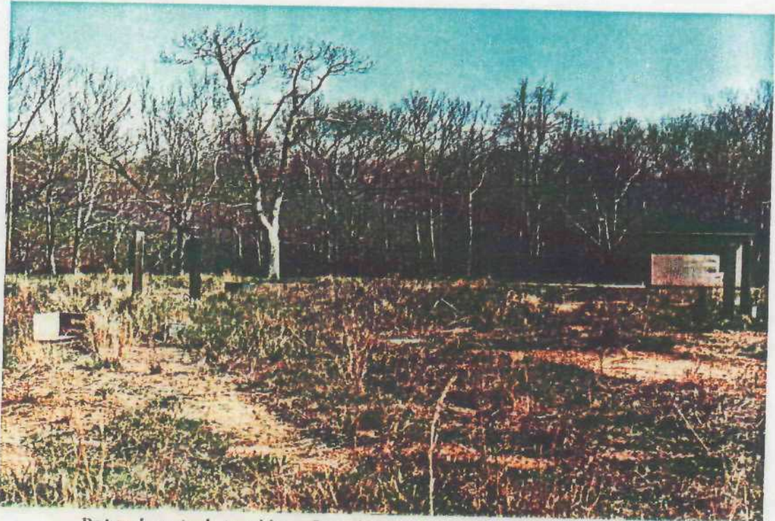
Deteriorated trailer-foundations with utility posts, deteriorated bus-stop shelter in background.
