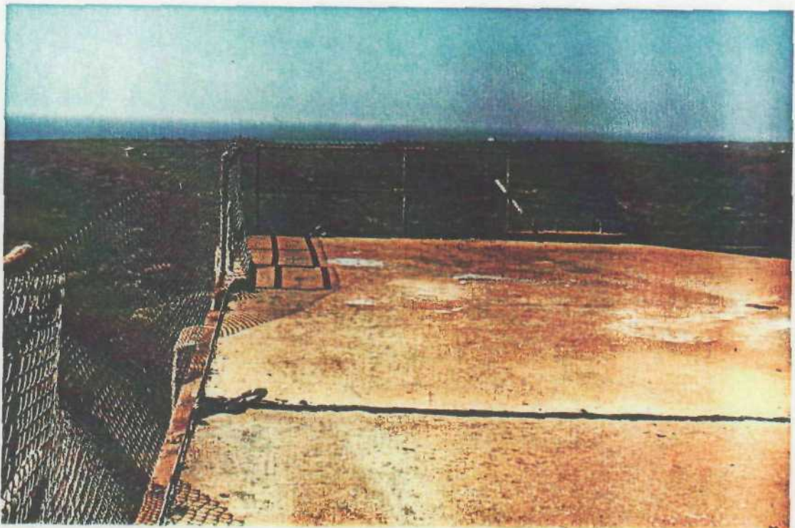
Deteriorating fence on top of radar tower #P-201.
