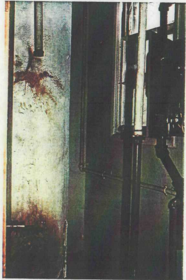
Deteroration inside bldg. #T-1.
