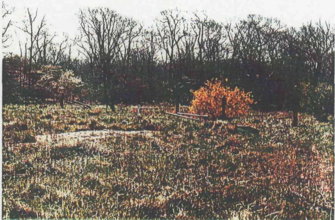
Deteriorated trailer foundations with utility posts.
