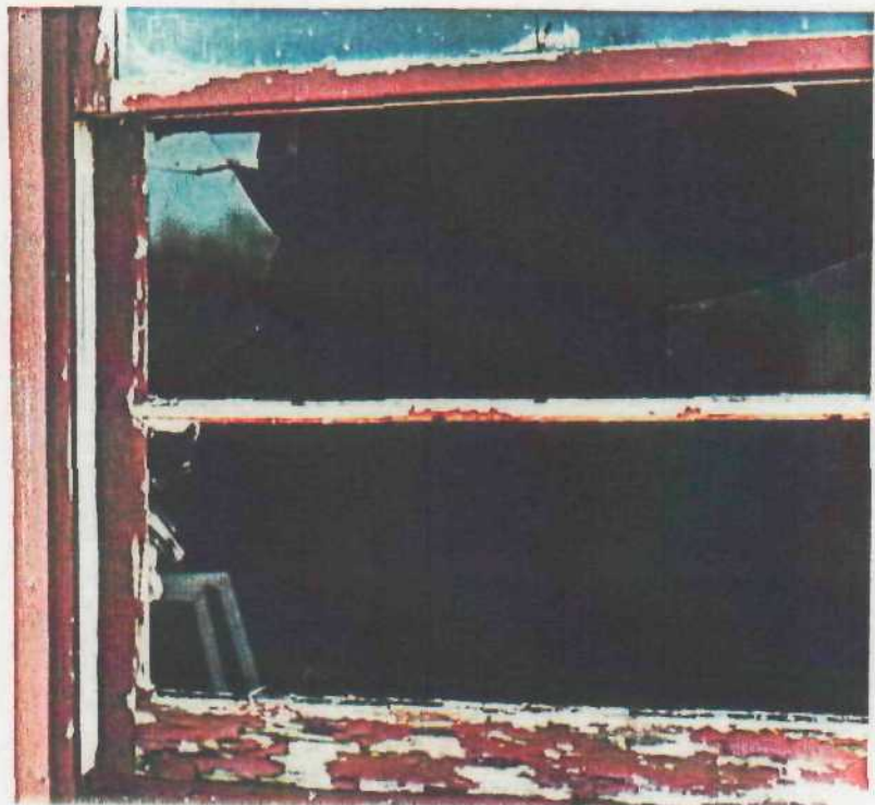
Broken glass in 2.5 foot high window of bldg. #P-119.
