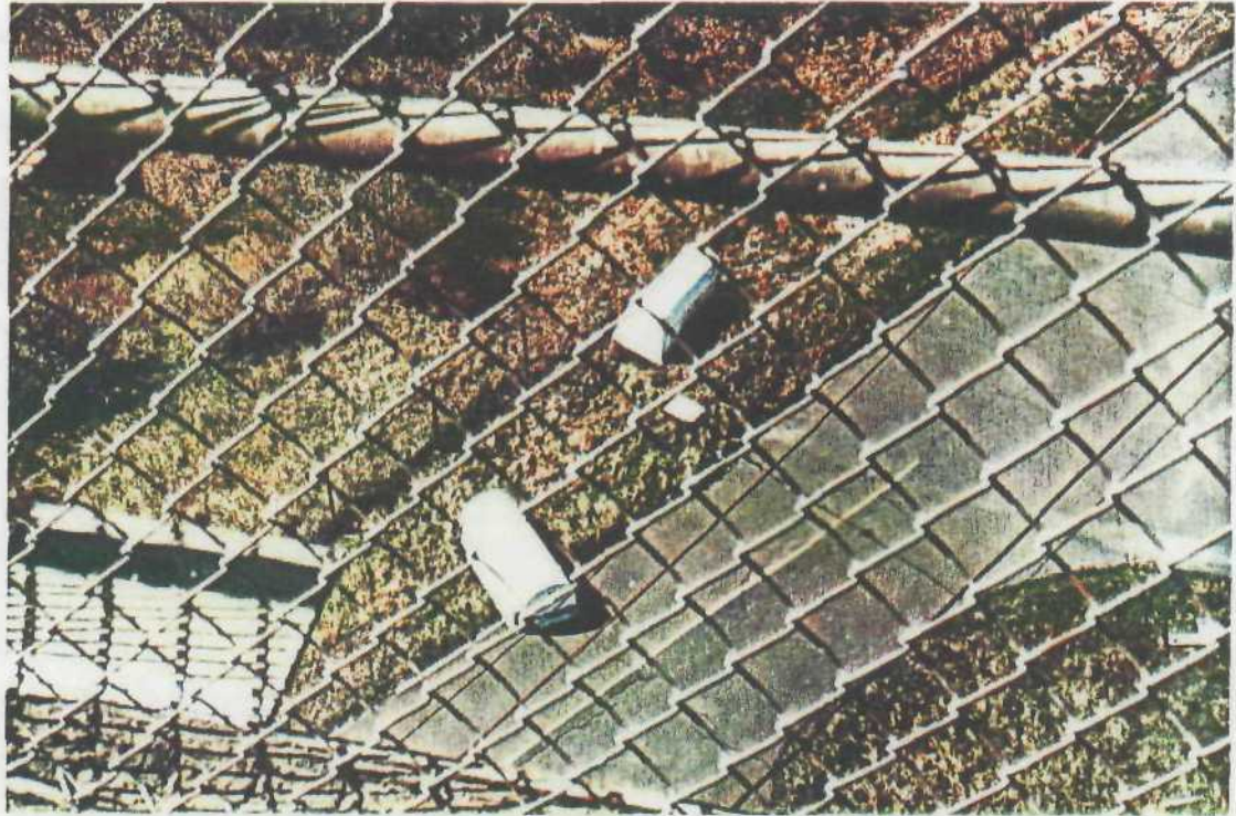
Two-six foot long generator covers, removed and thrown from roof of radar tower #P-201 probably by vandals.
