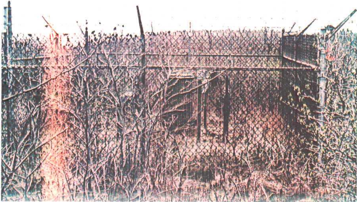
View of transformer and cage behind weather station (Bldg. #P-104).
