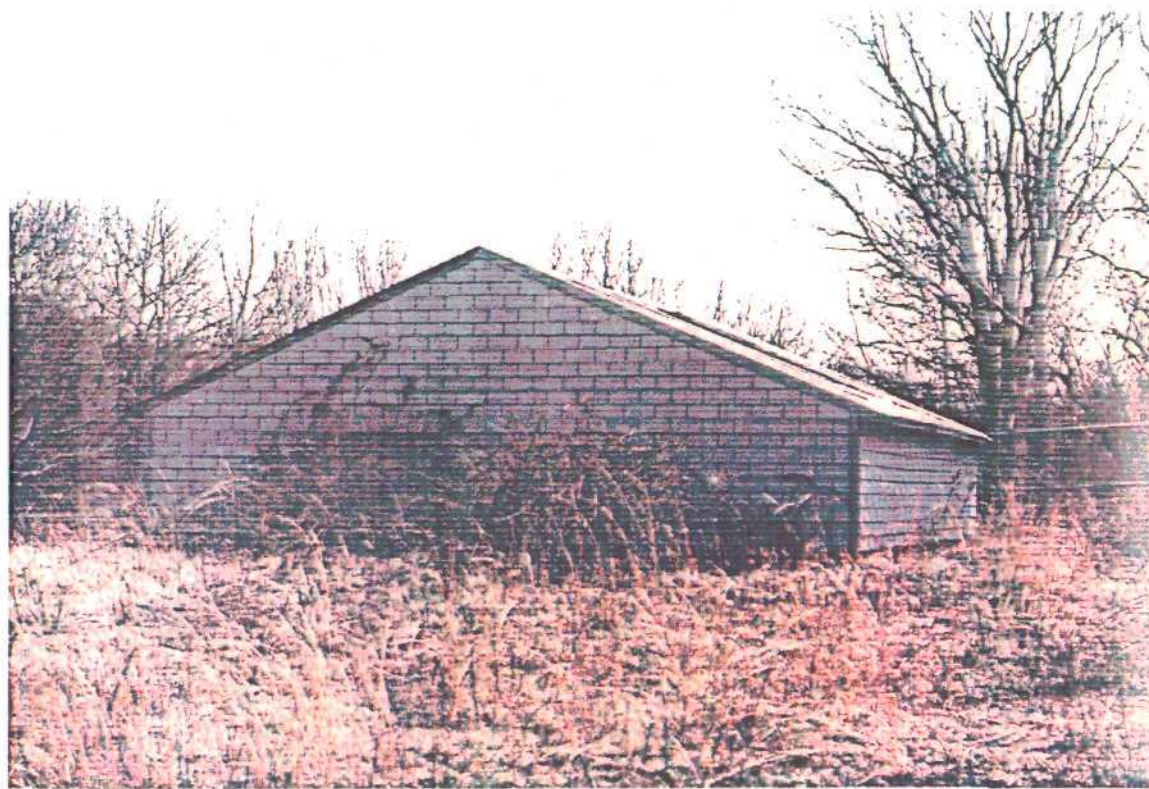
Portion of sewage treatment plant.
