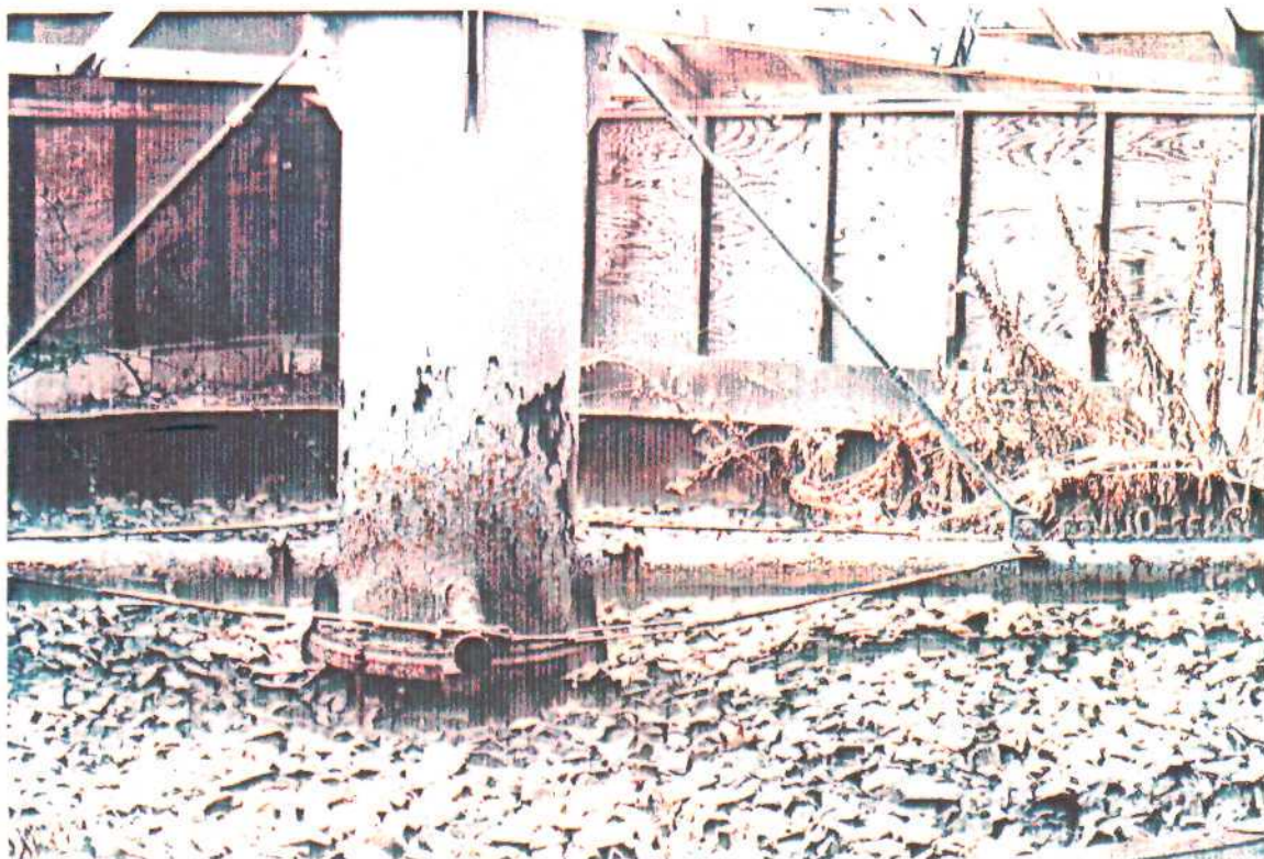
Portion of sewage treatment facilities.
