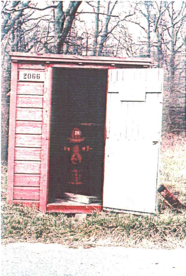
Fire hydrant inside of hose house (Bldg. #2066). Hydrant will not be removed.
