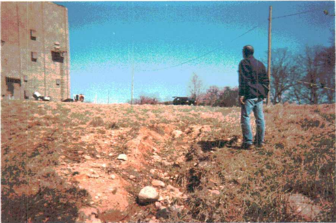
Photograph 4 - Erosional area south of the Radar Tower near SS-12.
