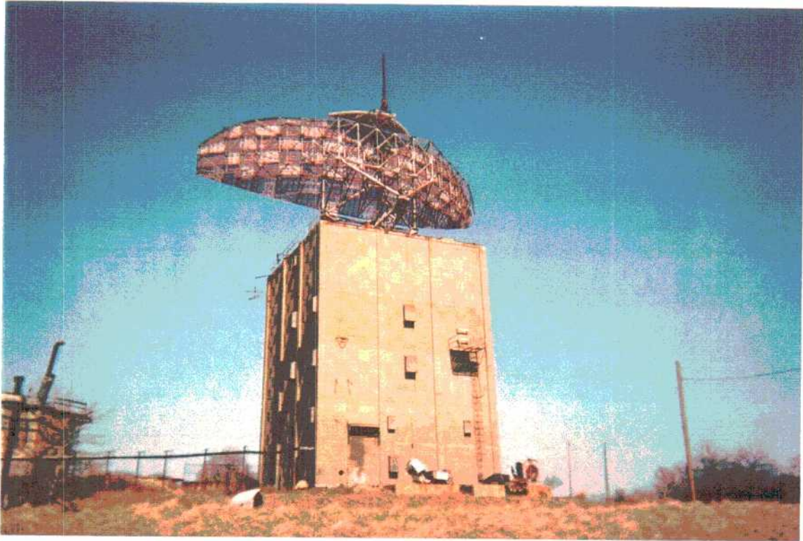
Photograph 7 - View of south side of Radar Tower. Sample SS-14 is located near the lower left corner of the building.
