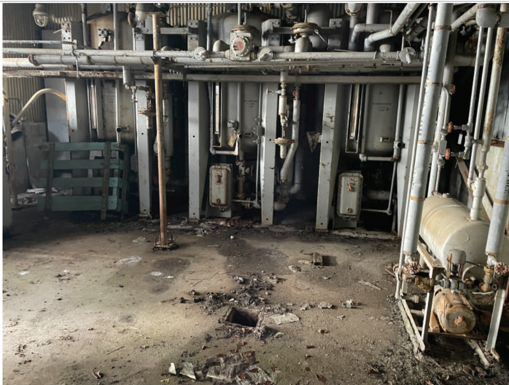
Floor Drain S-17
