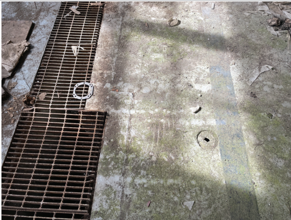
Floor Drain S-16
