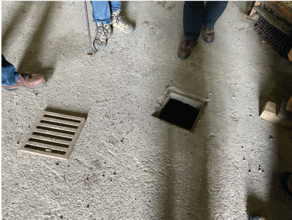
Floor Drain S-18
