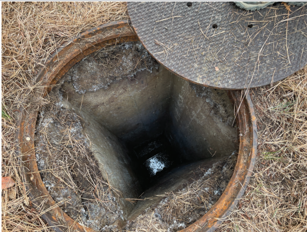
Septic Tank S-3
