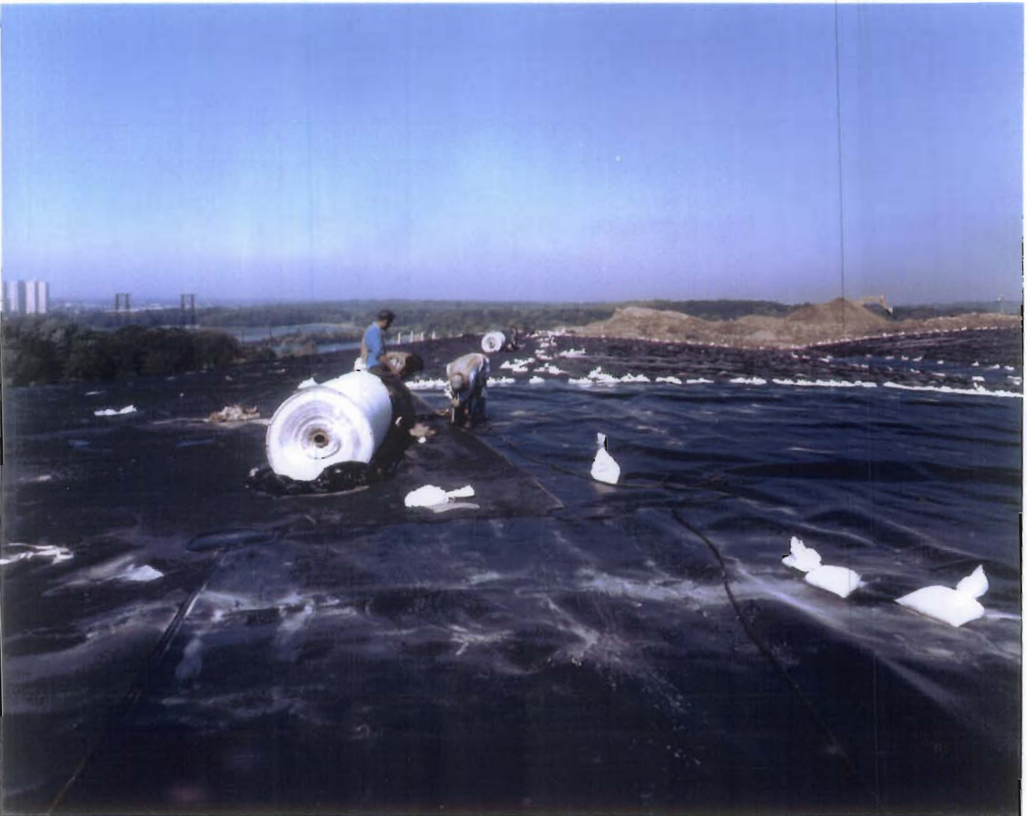
Photo No. 4. Seaming of Textured and Smooth HDPE Geomembrane at Top of Landfill (September 27, 1995)
