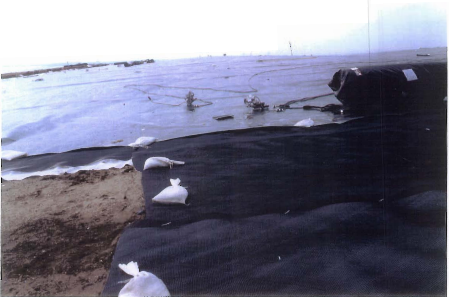
Photo No. 3. Installation of Smooth HDPE Geomembrane at Top of Landfill (November 1, 1995)
