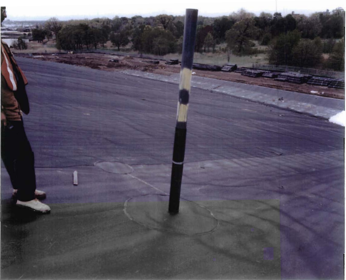
Photo No. 5. Detail of LFG Vent Boot. (May 11, 1995)
