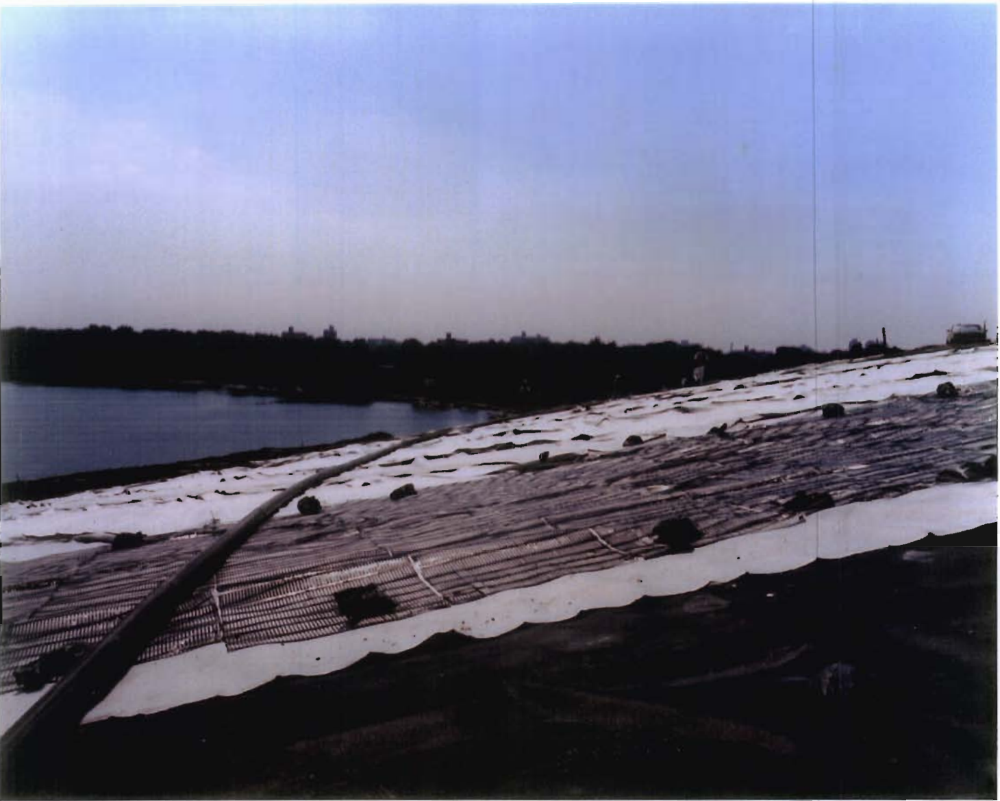
Photo No. 8. LFG Collection Pipe Installation over Geocomposite Layer (with Geogrid Reinforcement). (August 1, 1995)
