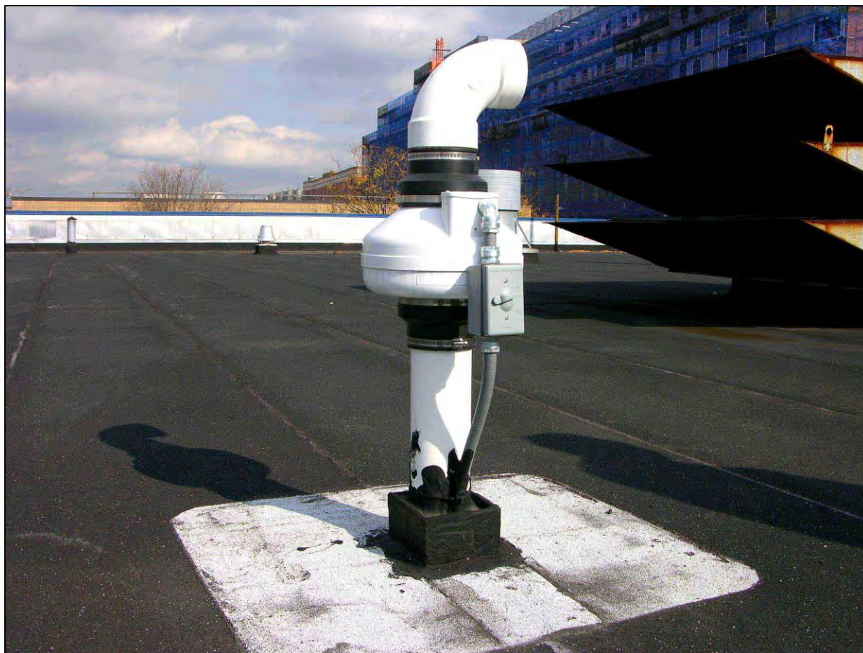
One of two sub-slab depressurization system vacuum fan units installed on the roof
