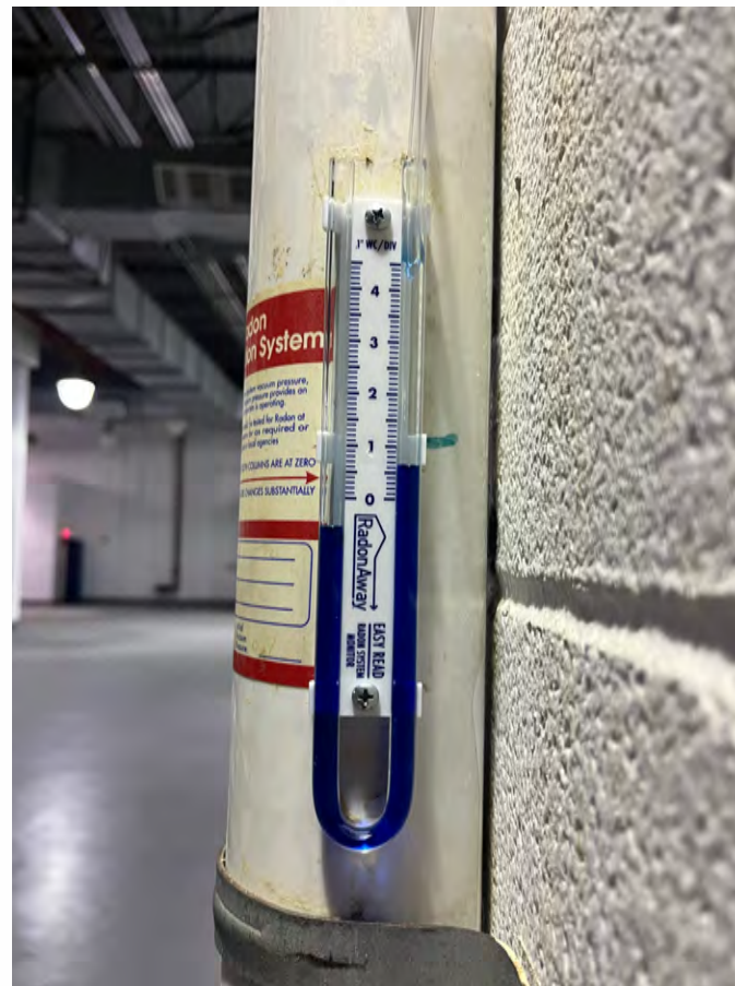
Sub-slab depressurization system vacuum indicator gauge attached to Eastern PVC riser
