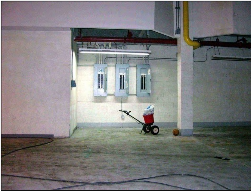
The sub-slab depressurization system circuit breaker is located on the center panel outside the boiler room
