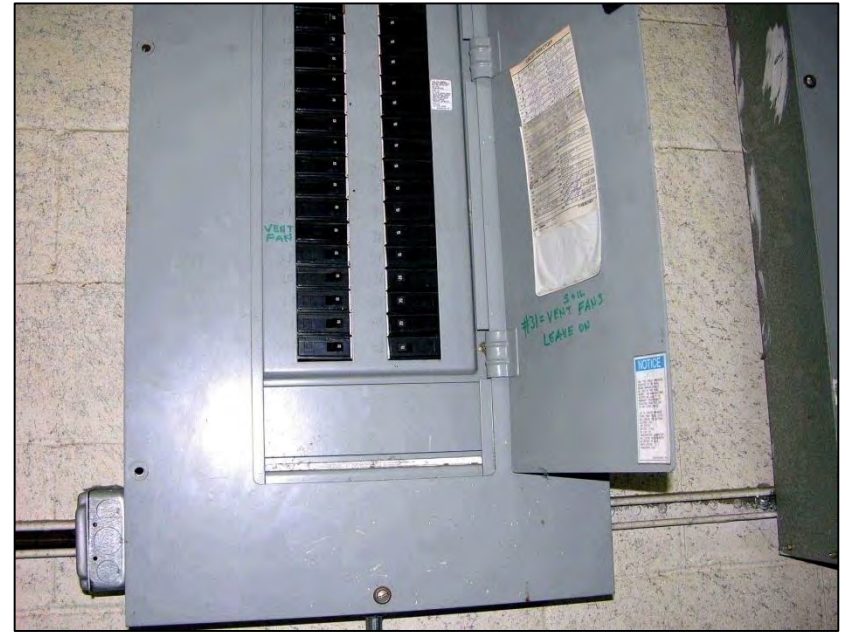
The sub-slab depressurization system circuit breaker is number 31, adjacent to the green markings on the panel
