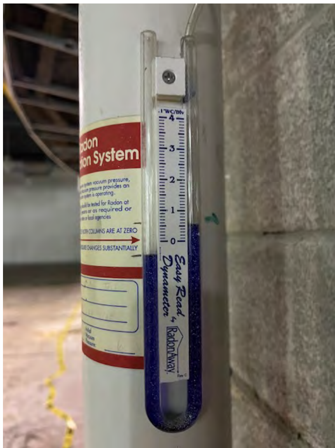
Sub-slab depressurization system vacuum indicator gauge attached to Western PVC riser
