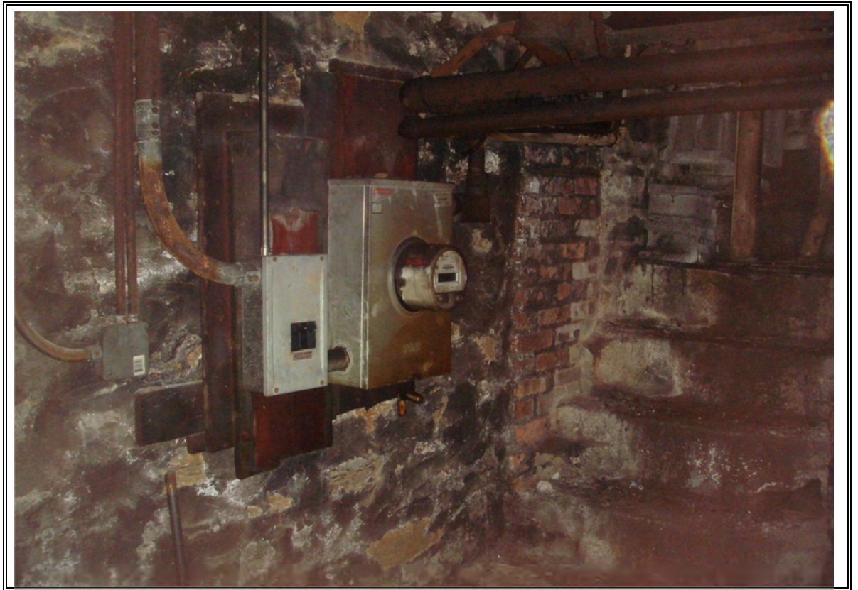
Photograph Number 9: Electric Meter
