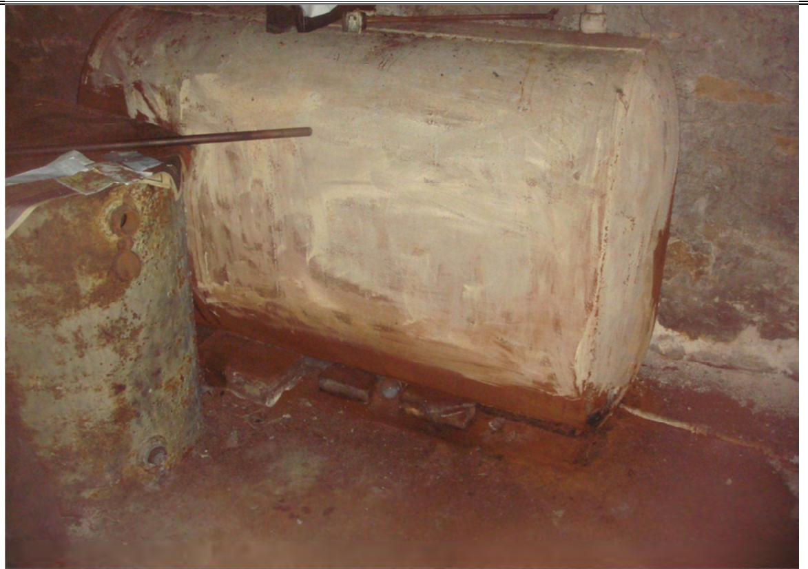
Photograph Number 8: 275 gallon fuel oil aboveground storage tank
