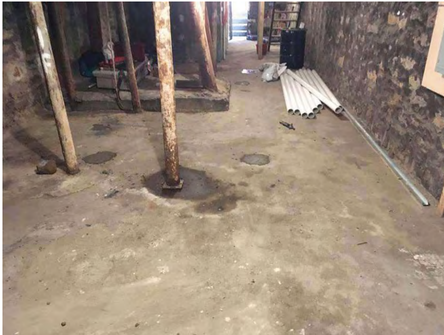
View of cellar at end of day, soil borings patched up with concrete
