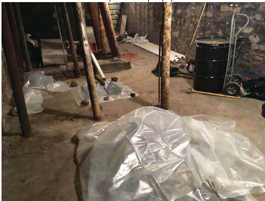
View of cellar at end of day. Pit and soil stockpile covered.
