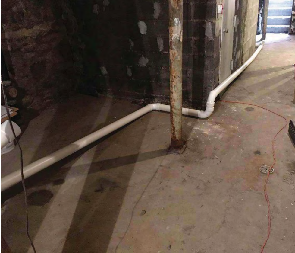
Additional view of cellar at end of day. PVC cut and fitted for hanging on 10-12-17
