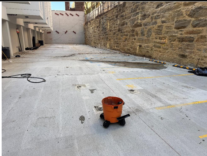
Photo 1: View of equipment removal in the northern portion of the Site, facing west.
