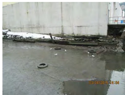
Looking at entrance of 11 th St. basin and bulkhead along North side of Pathmark building
