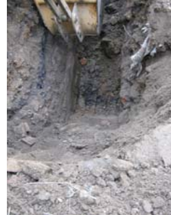
NATIONAL GRID EQUITY FORMER MGP SITE, BROOKLYN NY PLAN - 254 MASPETH AVENUE (REVISED) PREDESIGN INVESTIGATION ACTIVITIES (254 MASPETH AVENUE AND REMEDIAL INVESTIGATION ACTIVITIES (254 MASPETH AVENUE) FIGURE - 4
