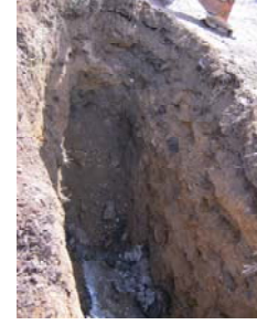
NATIONAL GRID EQUITY FORMER MGP SITE, BROOKLYN NY ENV WORK PLAN - 254 MASPETH AVENUE DATE: 12/22/2011 DRAWN: BUNQUELL/DSE PRE-DESIGN INVESTIGATION ACTIVITIES (252 & 254 MASPETH AVENUE) AND REMEDIAL INVESTIGATION ACTIVITIES (254 MASPETH AVENUE) FIGURE -4
