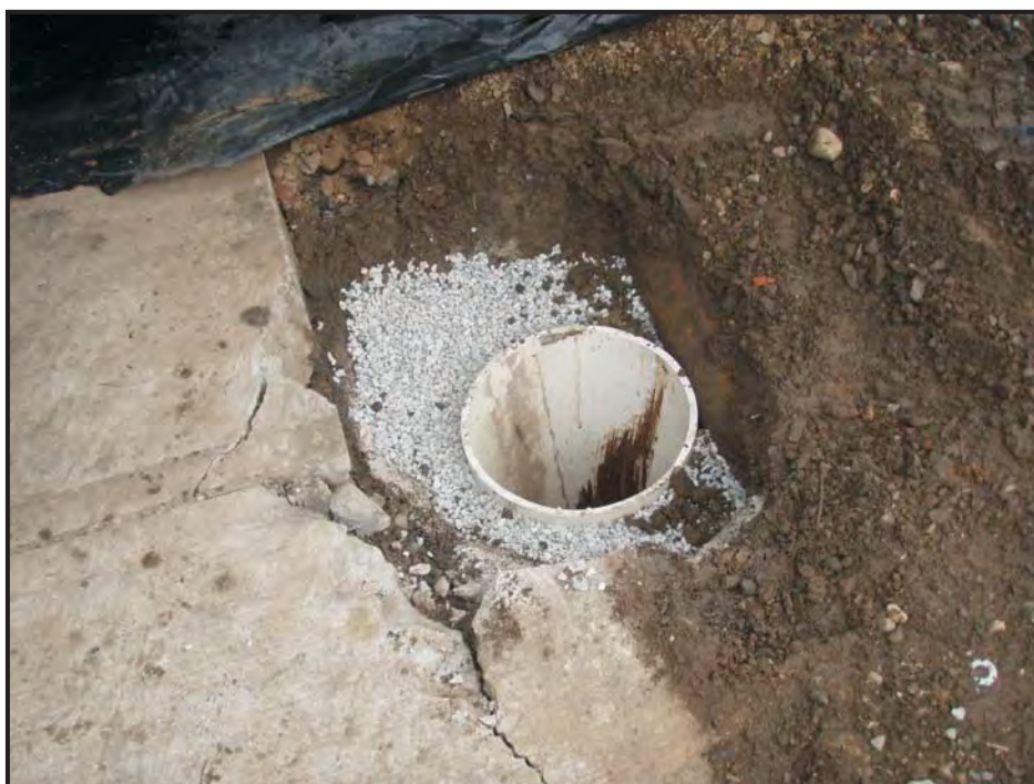
Photo 18: PVC casing plug for 24" inactive gas line.
