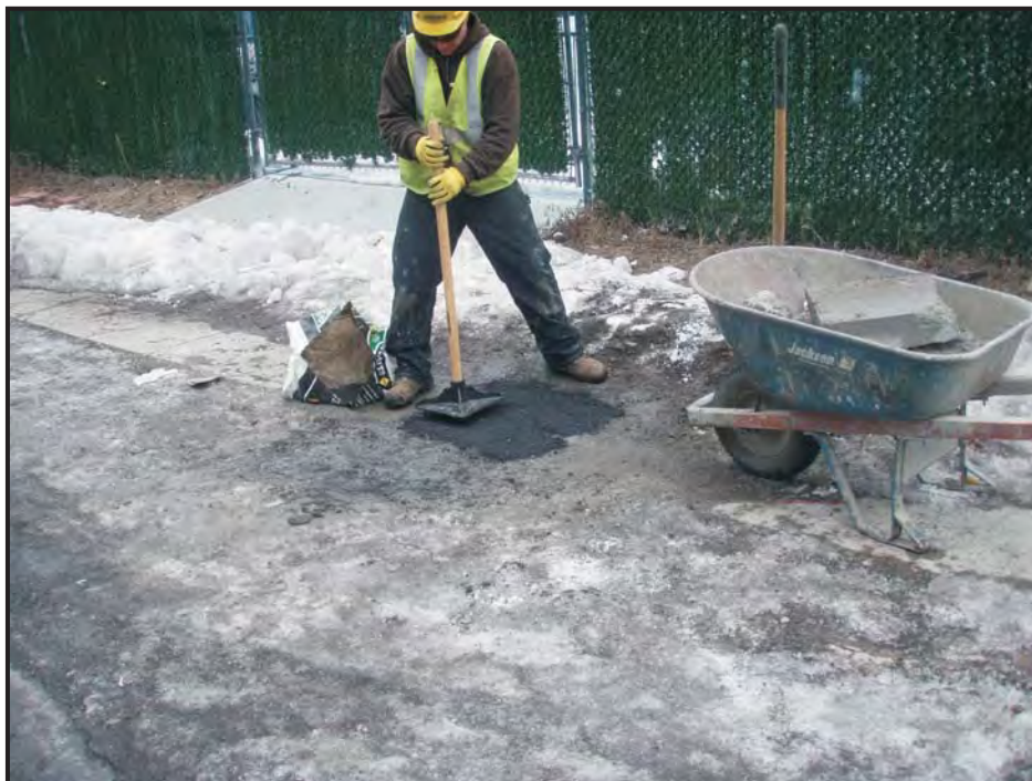
Photo 4: Asphalt patch over backfilled hole.
