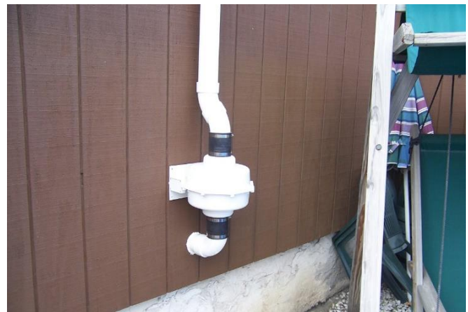
Typical example of a residential soil vapor mitigation system
