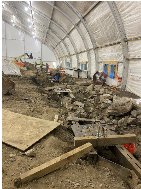
Photo 2: View of steel installation along exposed section of interior sheet pile wall, facing south.
