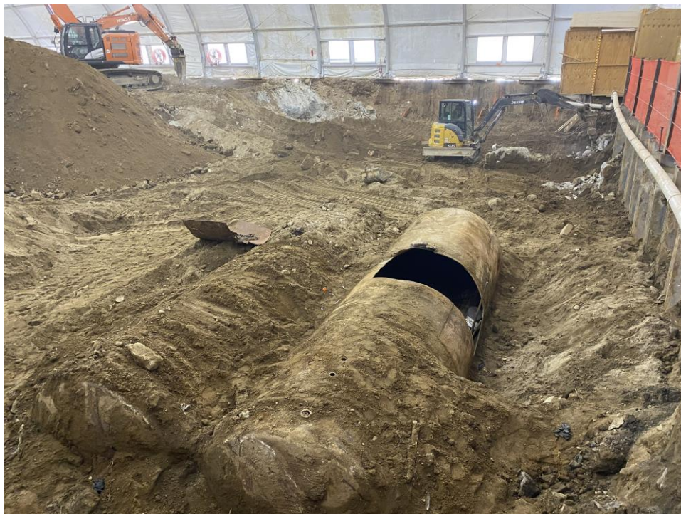
Photo 2: View of cleaning access cutout in uncovered tank within the enclosure, facing east.
