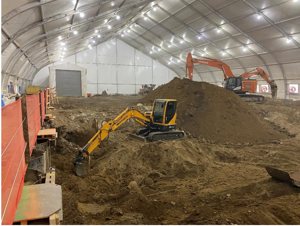
Photo 1: View of excavation and stockpile of soil from 0 to 6 ft bgs facing northeast.
