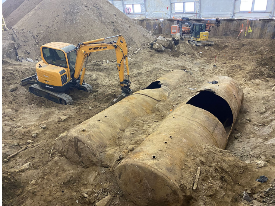
Photo 2: View of TK-6 & TK-7 within the enclosure, facing east.
