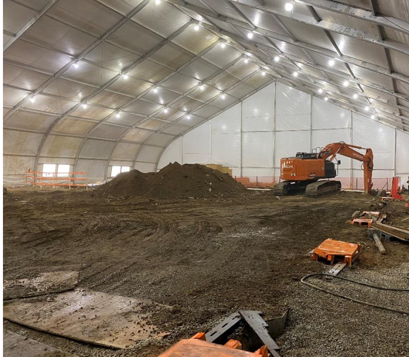
Photo 1: View of excavator stockpiling soil within the enclosure from 0 to 6 ft bgs.
