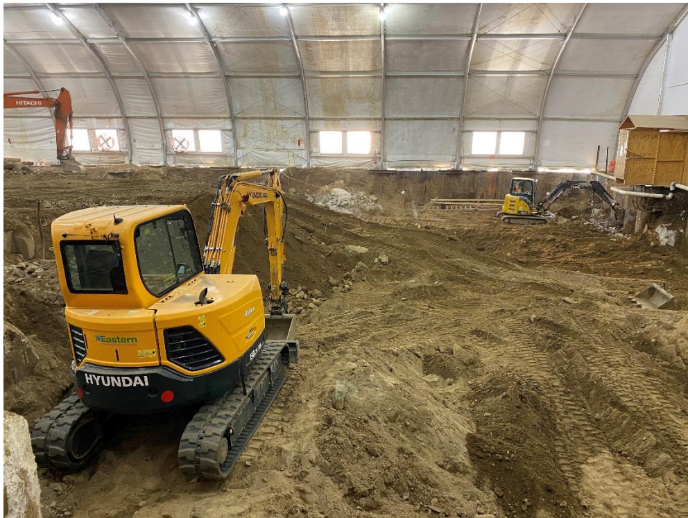
Photo 2: View of excavation on the southern portion of the Site in the enclosure.
