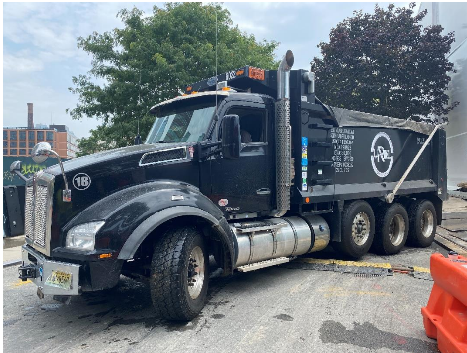
Photo 2: View of covered truck containing soil from 0 to 6 ft bgs exiting the enclosure after being washed.
