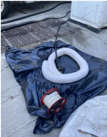
Photo 2: View of spill containment setup, interface probe meter and vac truck flexible hose inserted into RW-25.
