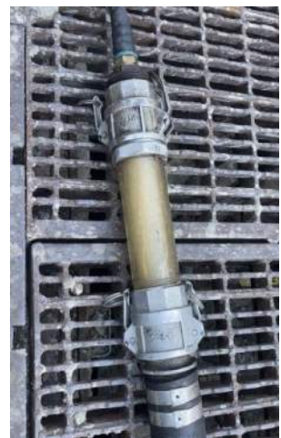
Photo 6: View of groundwater extraction passing through transparent pipe section of vac truck flexible hose.
