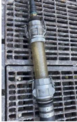
Photo 7: View of groundwater extraction passing through transparent pipe section of vac truck flexible hose.
