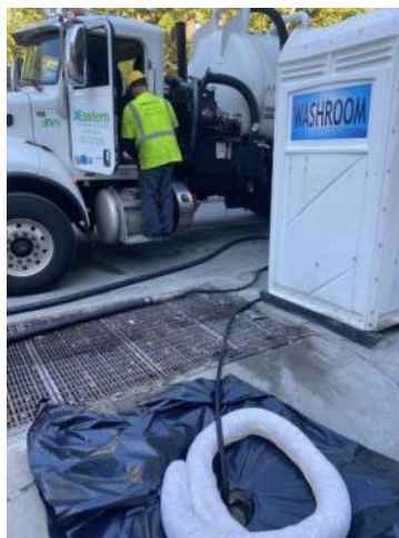
Photo 3: View of vac truck and environmental contractor personnel staged adjacent to RW-25.
