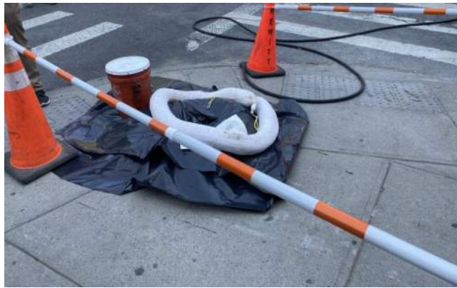
Photo 8: View of spill containment setup and pedestrian delineation at MW-26 on the southeast corner of Dupont and Franklin Street.
