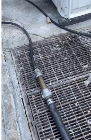
Photo 4: View of transparent pipe section of vac truck flexible hose.
