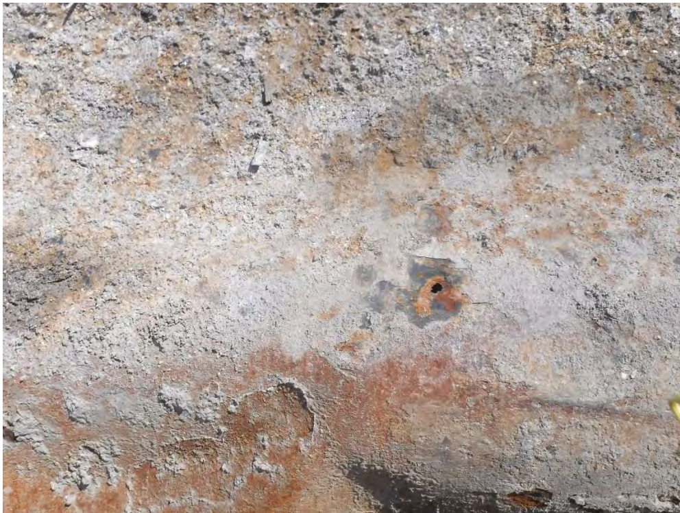
Photograph No. 4: View of a corrosion hole along the sidewall of the UST.
