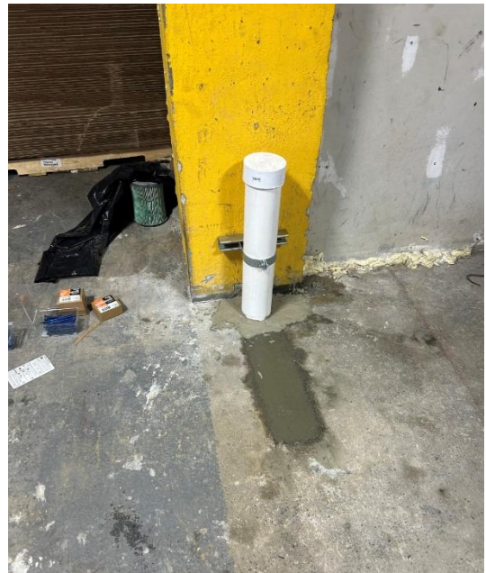
SP-4 installed along interior column in Linwood Street warehouse along wall separating the two warehouse spaces
