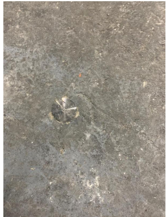
Vacuum monitoring point (VMP) finished condition (typical)
