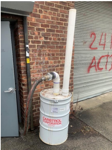
Pilot test effluent discharge point along Linwood Street sidewalk through VPGAC drum
