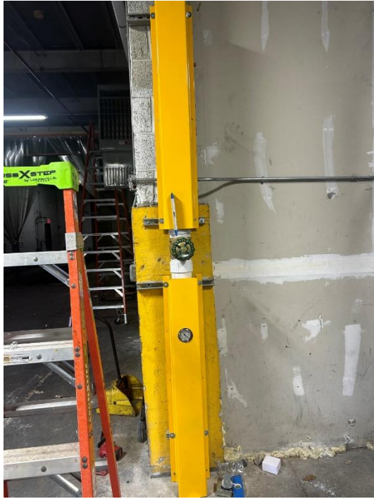
Steel guard installed around SP-4 with gate valve, vacuum alarm, and vacuum gauge accessible
