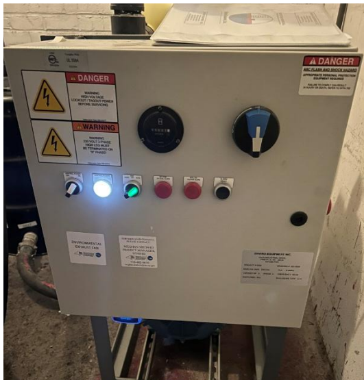
Control panel under normal operating conditions (NYSDEC PM contact information labels visible in bottom left corner)
