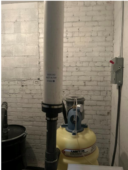
Circuit switch located adjacent to blower (seen on the right)
