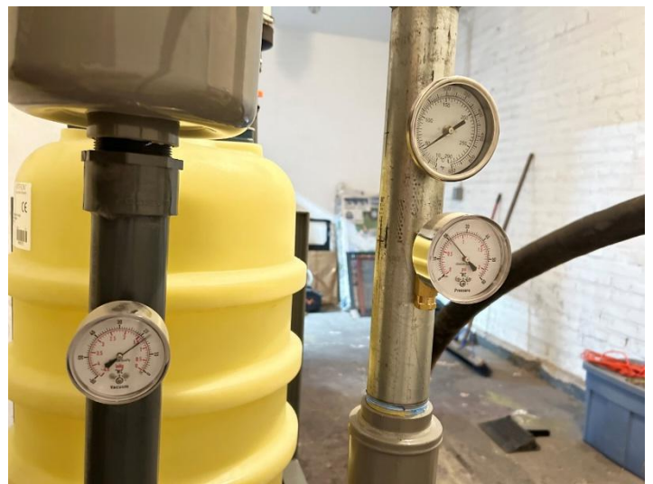
Vacuum (left), pressure (bottom-right), and temperature (top-right) gauges on influent and effluent piping located on backside of blower
