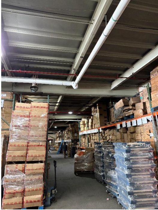
Pipe insulation and directional arrows installed to riser within Essex Street warehouse
