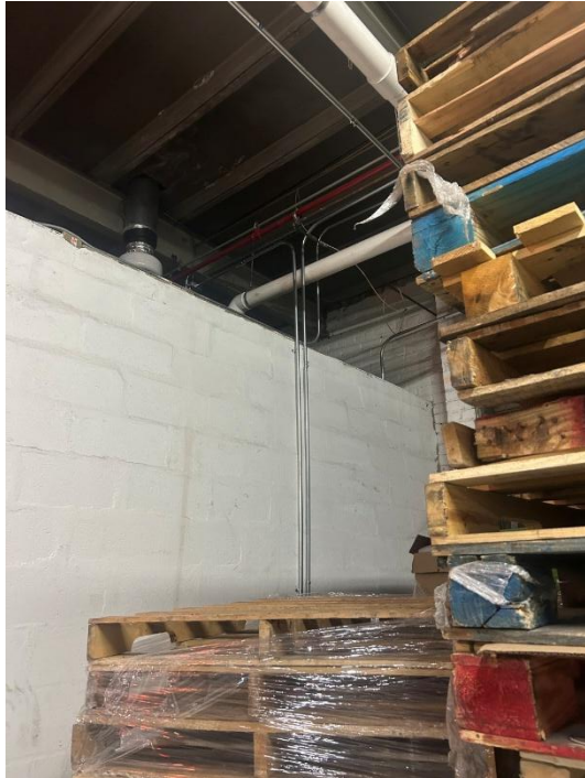
Piping routes through the ceiling of storage room to blower
