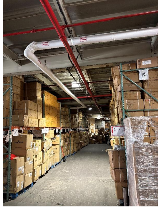
Pipe insulation and directional arrows installed to riser within Essex Street warehouse
