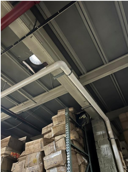
SP-3 piping runs along ceiling towards Linwood Street warehouse (piping runs southwest)
