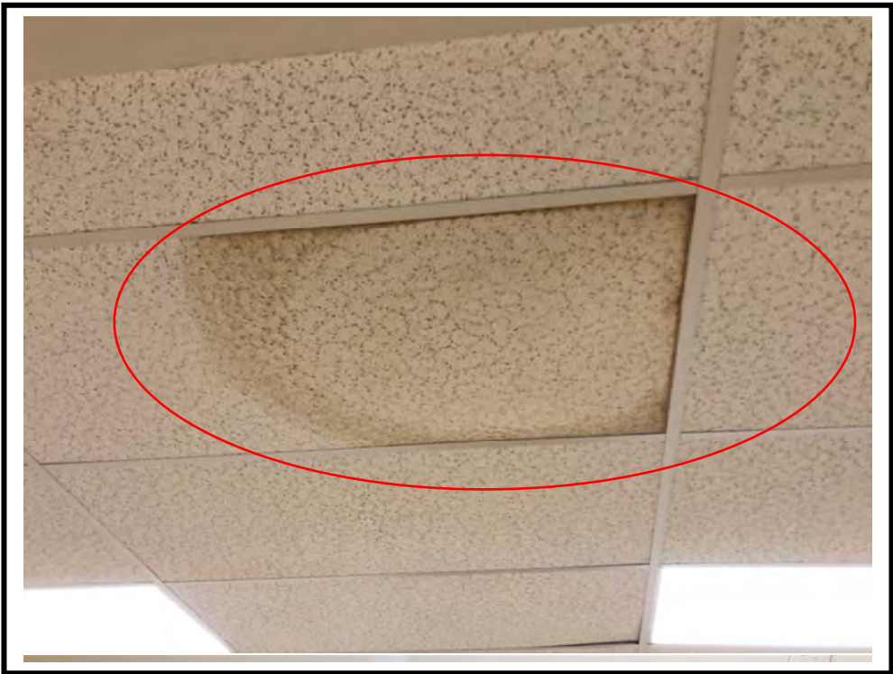
PHOTO LOCATION: Depicts water staining on the ceiling.
