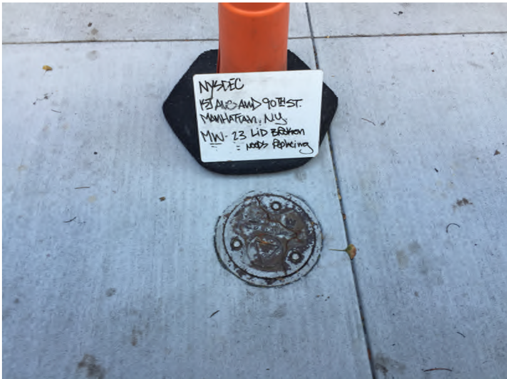
Photograph 18: Condition of MW-23 – Lid broken and needs replacement
