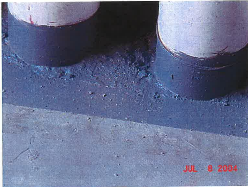
Photograph 3: Close-up view of sealed concrete around risers for soil vapor extraction system laterals in northeastern portion of Outer Warehouse.
