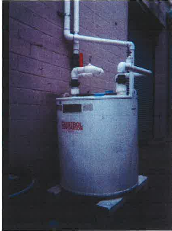
Photograph 9: View of G-4 GAC unit (primary).
