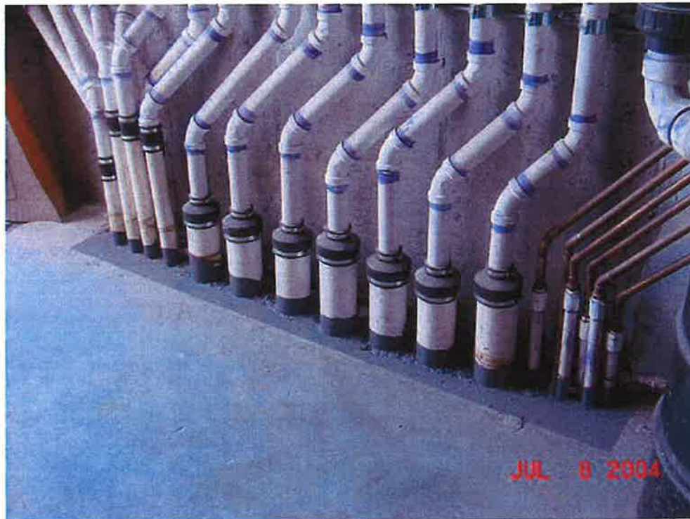
Photograph 2: View of sealed concrete around risers for soil vapor extraction system laterals in northeastern portion of Outer Warehouse.
