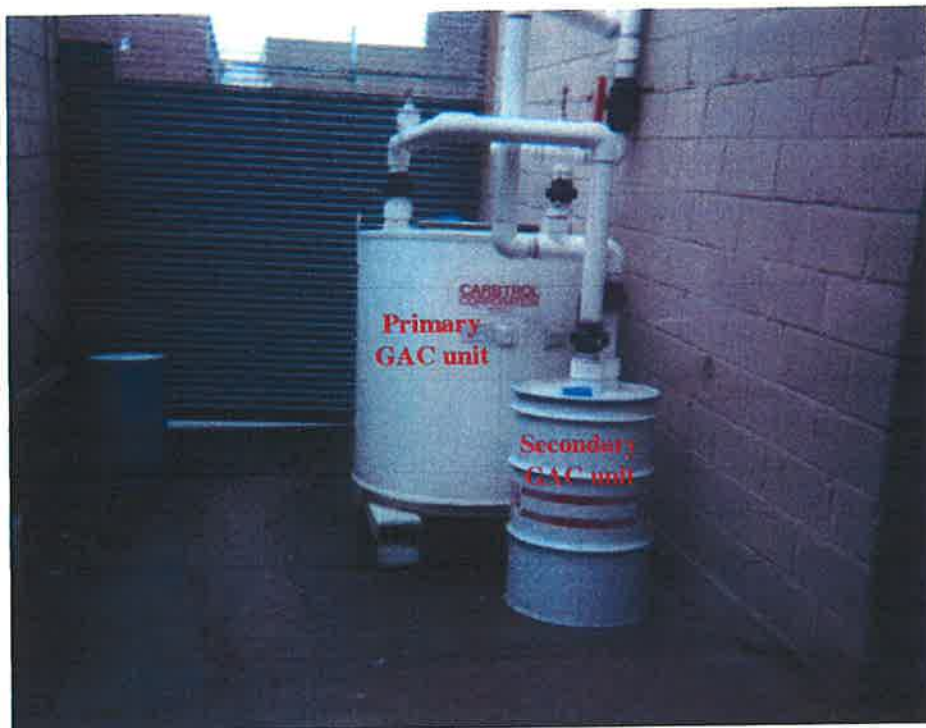
Photograph 11: View of GAC units in breezeway.
