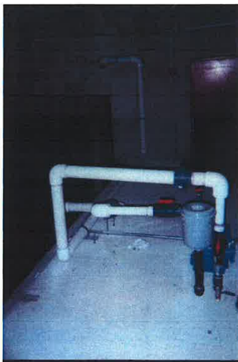
Photograph 4: Blower and piping to vent wells on roof of reactive vault.
