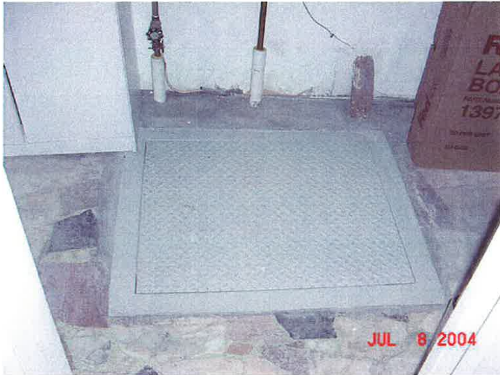
Photograph 5: View of sealed potential vapor migration pathway in office area.
