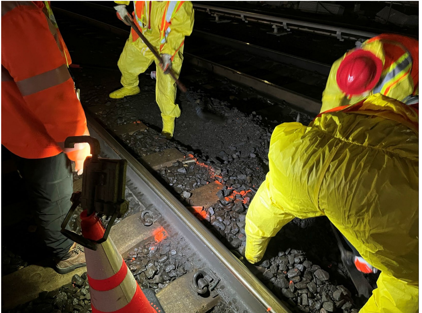
Photo 3: View facing northeast; Amtrak laborers digging to 2 ft bls for LLS-11A_N samples
