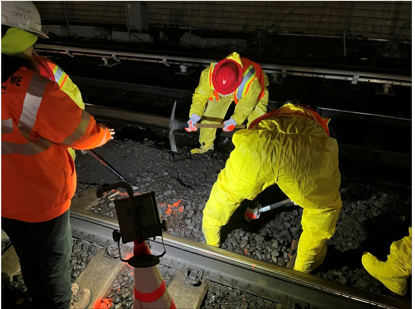
Photo 2: View facing east; Amtrak laborers digging to 2 ft bls for LLS-11A_S samples.
