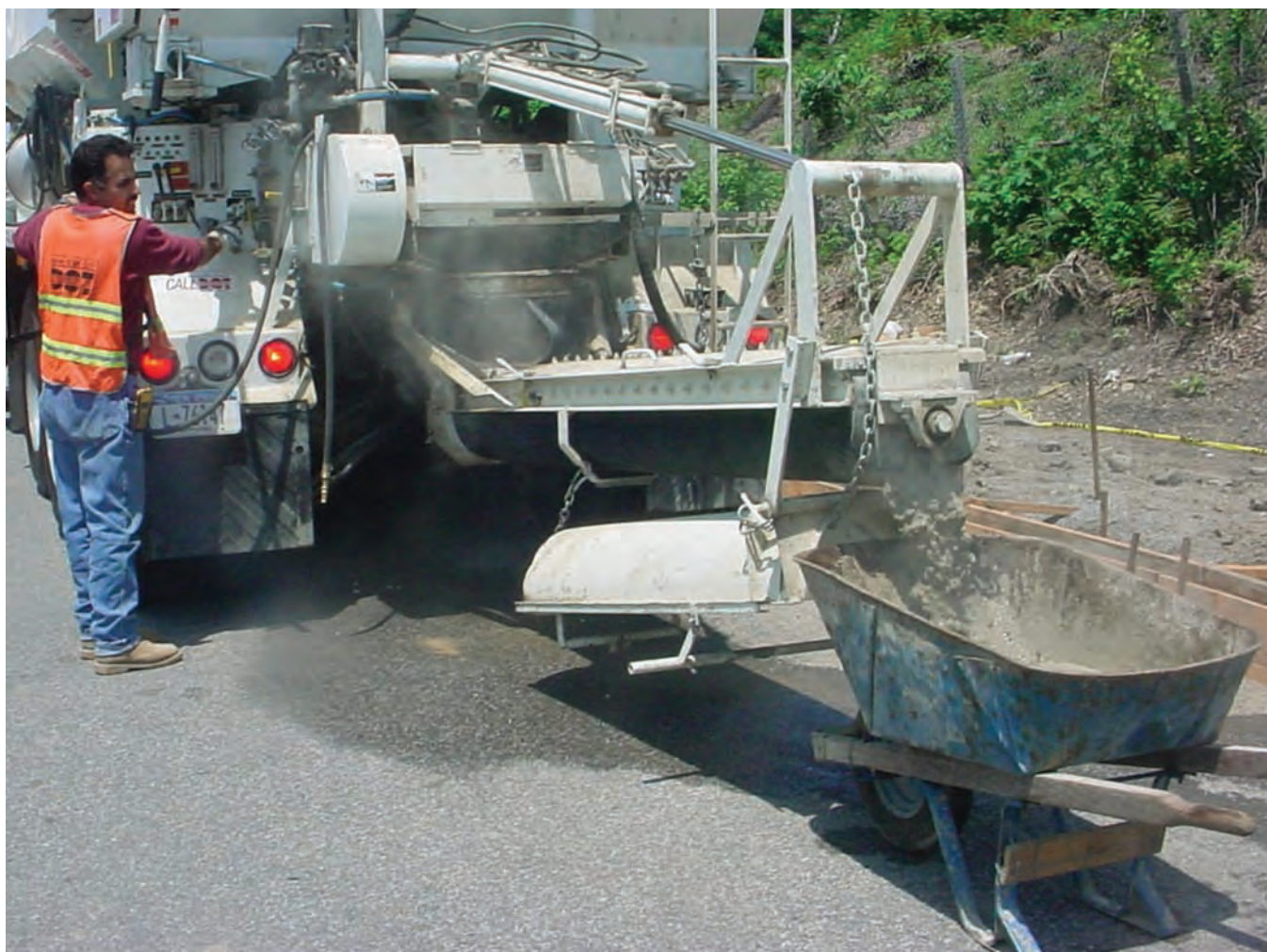
All work within the street requires a NYC DOT permit to minimize construction impacts.
