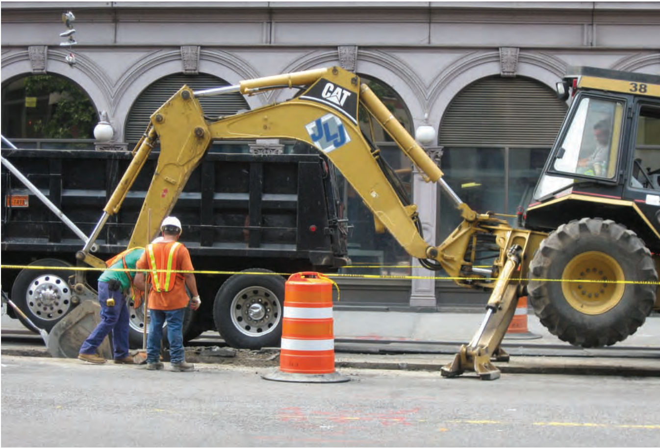
Street work at Third Avenue and Saint Marks Place, Manhattan as part of a larger Cooper Square area reconstruction project.
