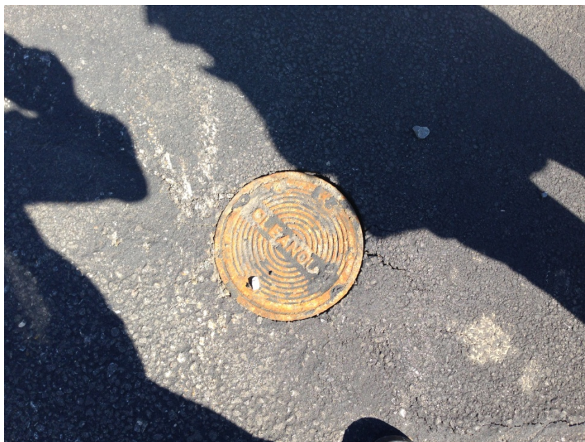
Photo 2: Cleanout Port (Facing North)
