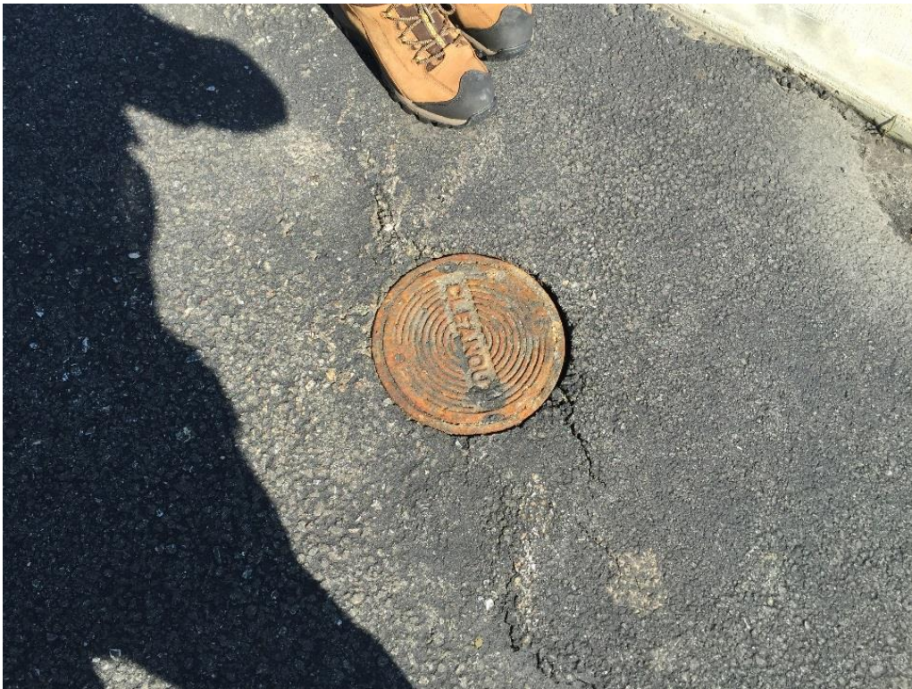
Photo 2: Cleanout Port (Facing North)
