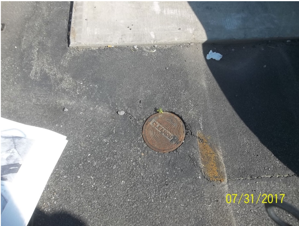
Photo 2: Cleanout Port (Facing North)
