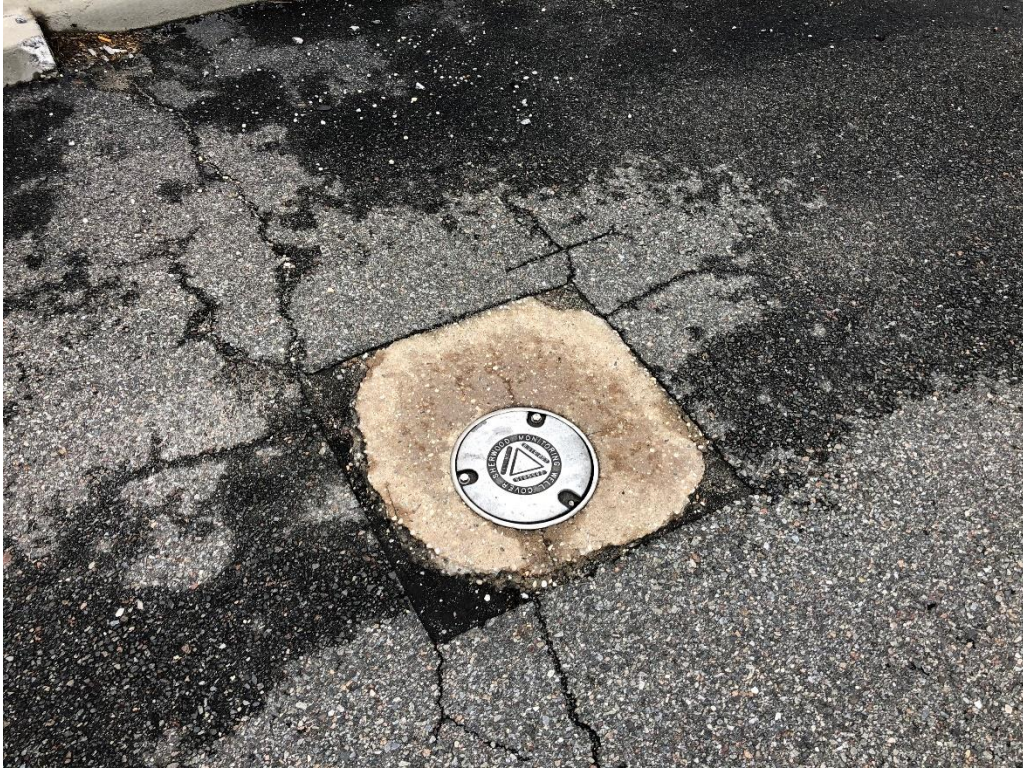
Photo 3: Monitoring Well MW-9 (Facing Southeast)
