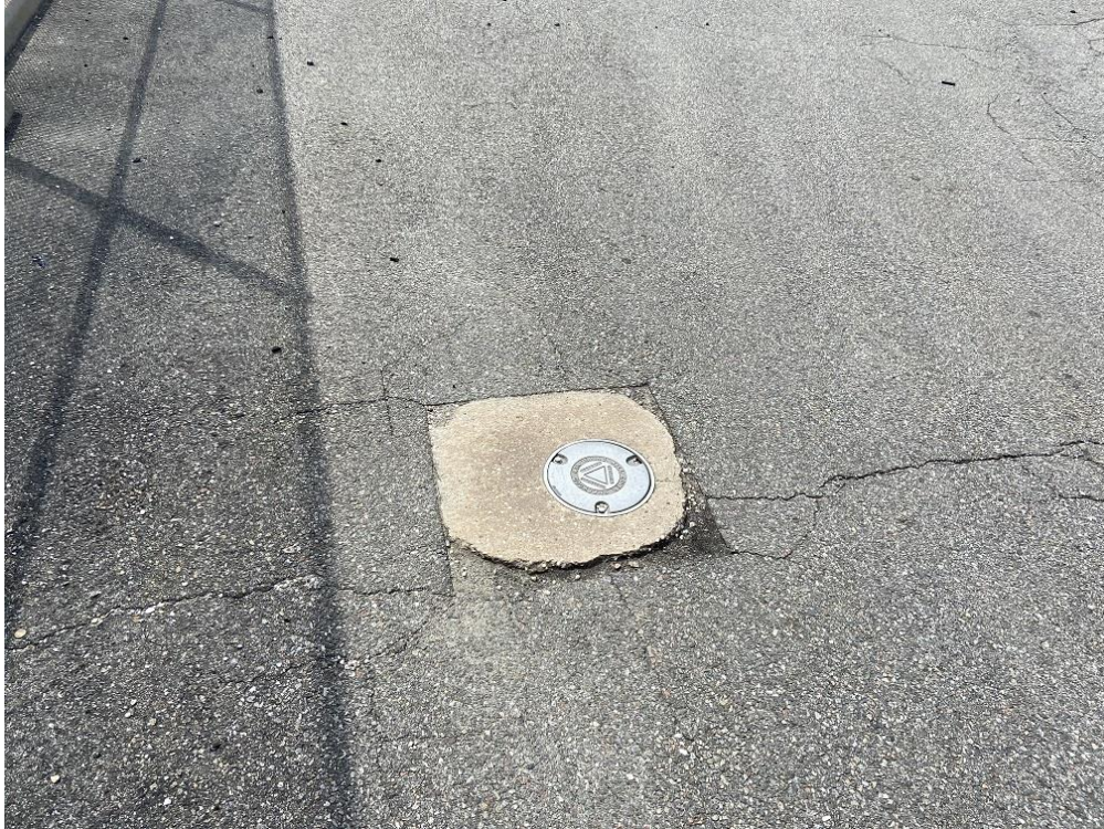
Photo 3: Monitoring Well MW-9 (Facing Southeast)
