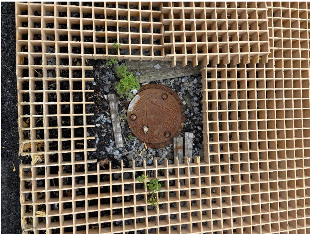
Photo 4: Monitoring Well MW-15 (Facing South)
